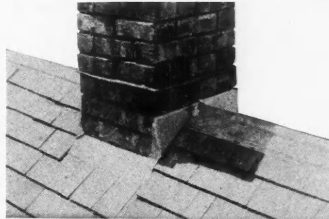
Chimney Water Guard in Use
