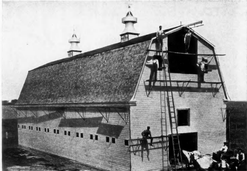
Reliable Scaffold Brackets in Use by Barn Builder John Willmann, Oriska, N. Dak.
