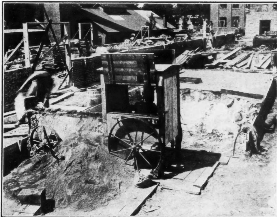
View Showing the Method of Preparing Mortar as Used by the Byers Construction Company of Kalamazoo, Michigan.
