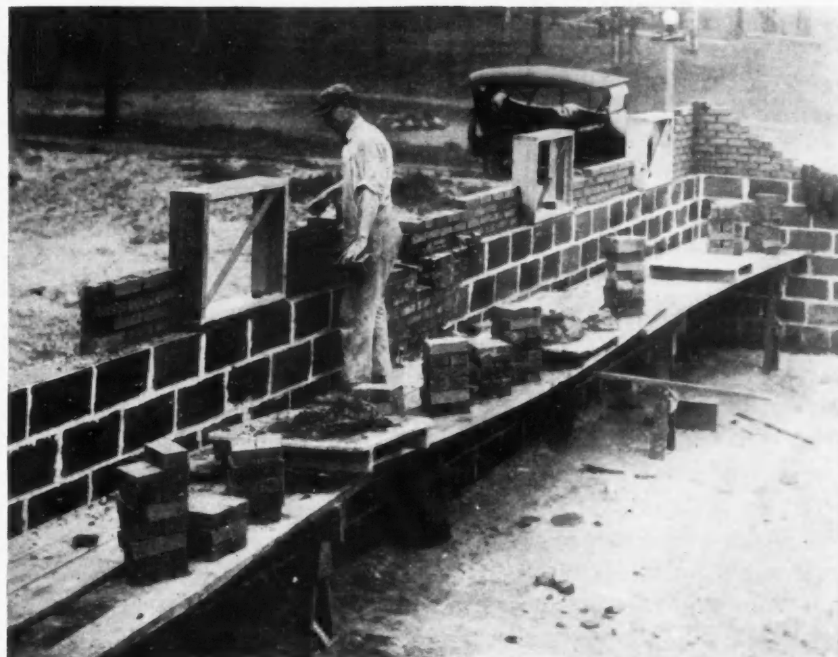
Combination Face Brick and Hollow Tile Wall in Course of Construction, Showing Setting of Basement Window Frames.
