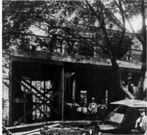
The Work Under Way. Framing Brought Out to the Sidewalk Line and First Floor Cleaned Out to Form Two Store Rooms.
