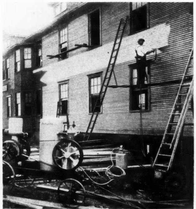
By the Use of This Portable Equipment, Paint Is Forced Thru the Tubing and Sprayed on the Wall by Compressed Air.
