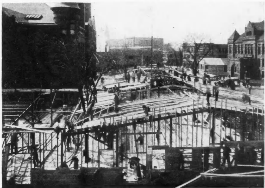
At 10 a.m. Flooring Nearly All Down, Sheeting Mostly on, a Good Start on the Siding. The Gap at the Left Was Strictly According to Schedule. The Men Working on the "L" Began at the Other End and Worked Toward the Main Section in Order to Make it Easier to Fit the Truss Where the Parts Join. Thruout the Day This Was the "Slow" Point.
