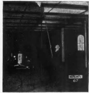
Speedy Process Eliminates Scaffolding. Most Economical System for Painting. Inaccessible Places Easily Reached.
