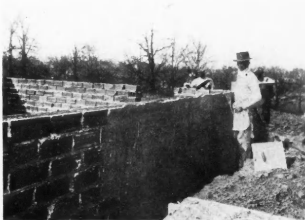
Many of the Alton Houses Have Tile Basement Walls. They Are Warm, Dry and Inexpensive.
