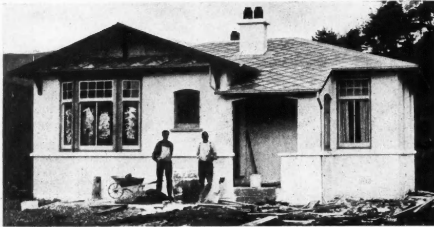
How They Build in New Zealand—A Concrete Hollow Wall Dwelling Built by an American Builder Reader at Upper Hutt, New Zealand.
