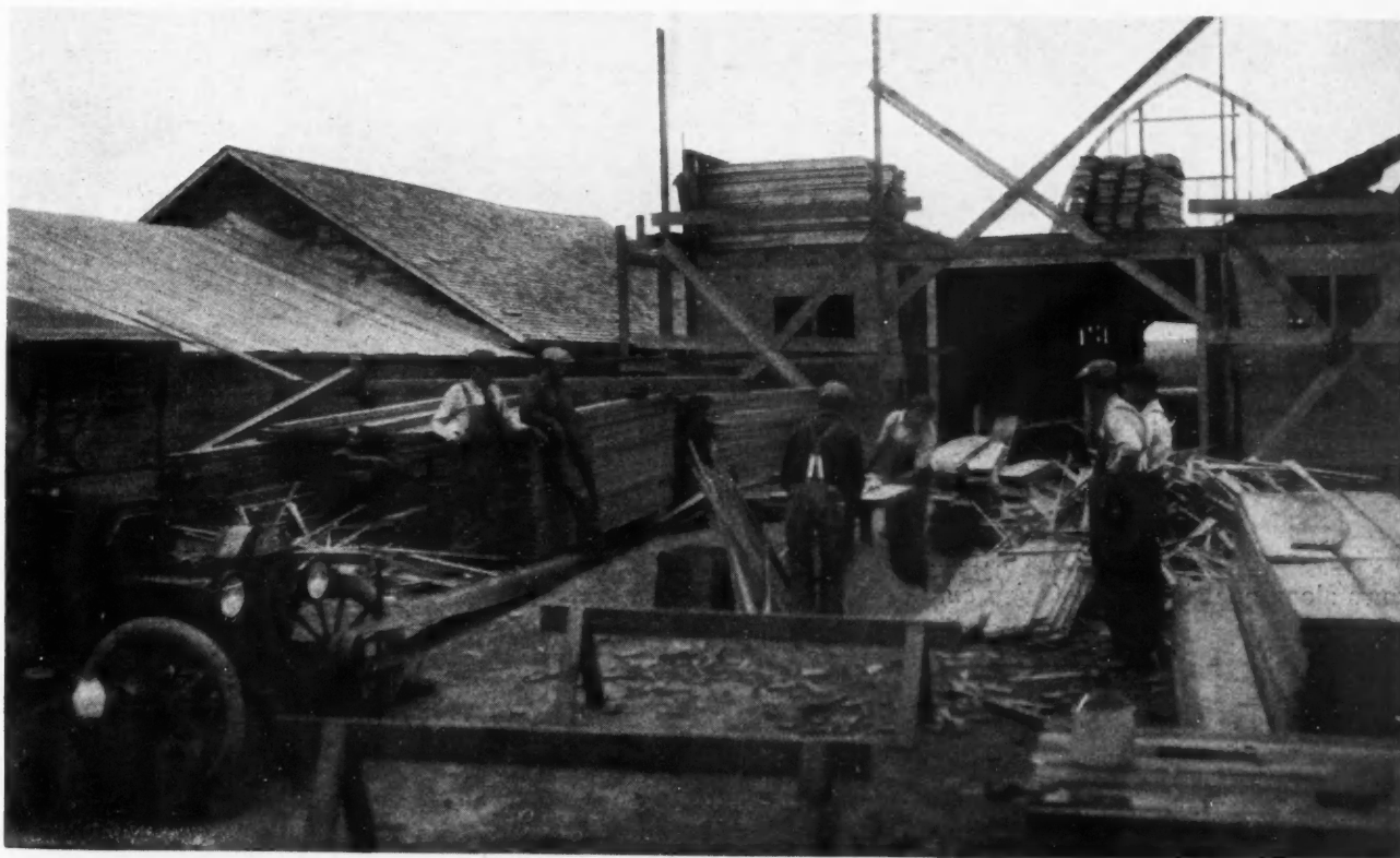
He Had a Power Saw Rig on the Job Ingeniously Hooked Up to His Ford Car for Power. Timbers Were Cut at a Great Saving.
