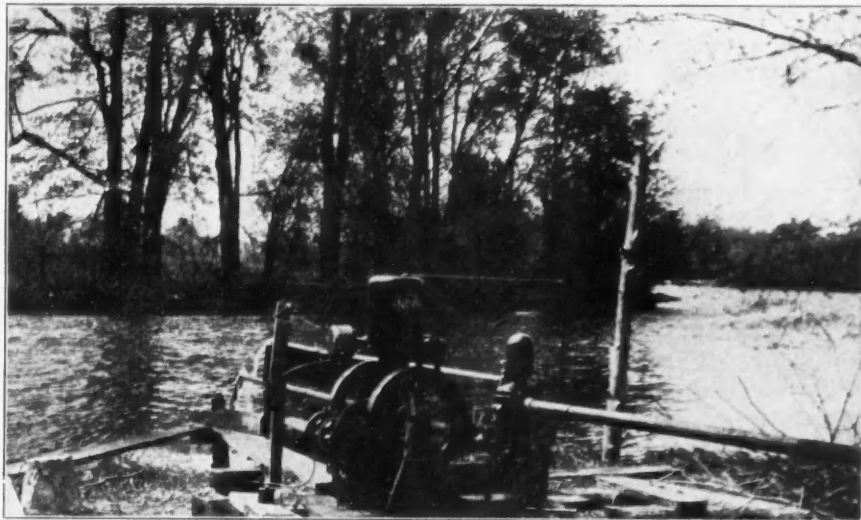
Pumping Outfit Taking Water from the Kalamazoo River, Near Battle Creek, Mich., and Delivering It to a Concrete Mixer on a Road Job Two Miles Away.
