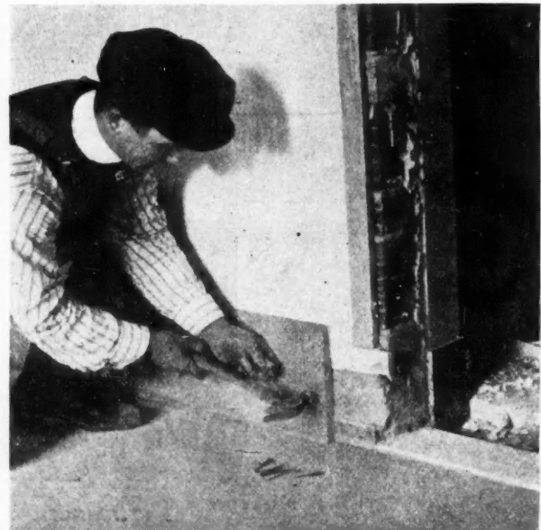
Nailing the Baseboard to Nailcrete. Note the Layers Between the Hollow Tiles Inserted so the Framework of the Door May be Conveniently Nailed Fast.
