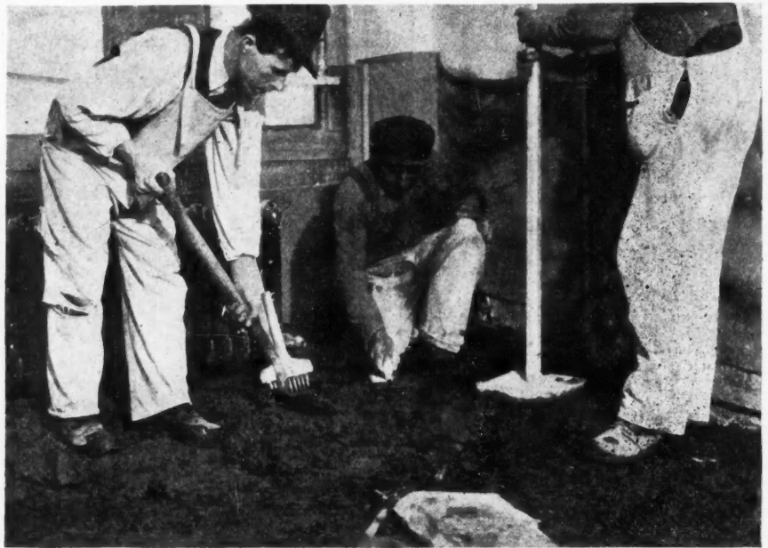
The Method of Laying Nailcrete. The Mixed Nailcrete is Wheeled in in a Barrow, Spread with a Shovel, Tamped Thoroughly, and Smoothed with a Leveler; After It Has Hardened a Smooth Surface Is Given It with a Polishing Machine.
