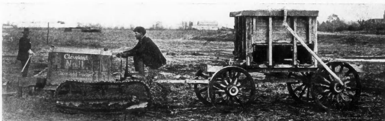
Caterpillar Tractors Carry Concrete Over a 450-Acre Site—Note Agitator in Mixed Concrete Vat to Prevent Settling of Concrete.
