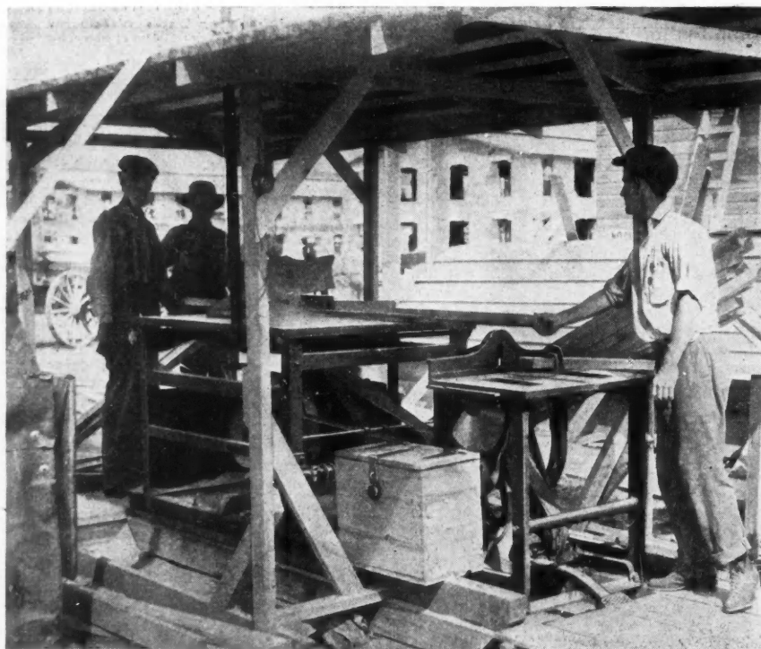
Cut-Off Saws and Portable Outfit Used by the A. Bentley & Sons Co. on Construction Work at Camp Sherman, Chillicothe, Ohio. This Equipment Transferred Part of the Woodworking Shop to the Job.
