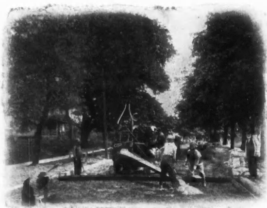
Cline & Boelens, Grand Haven, Mich., Contractors, Laid 600 Yards of Paving with This Mixer and a Crew of Eight Men.
