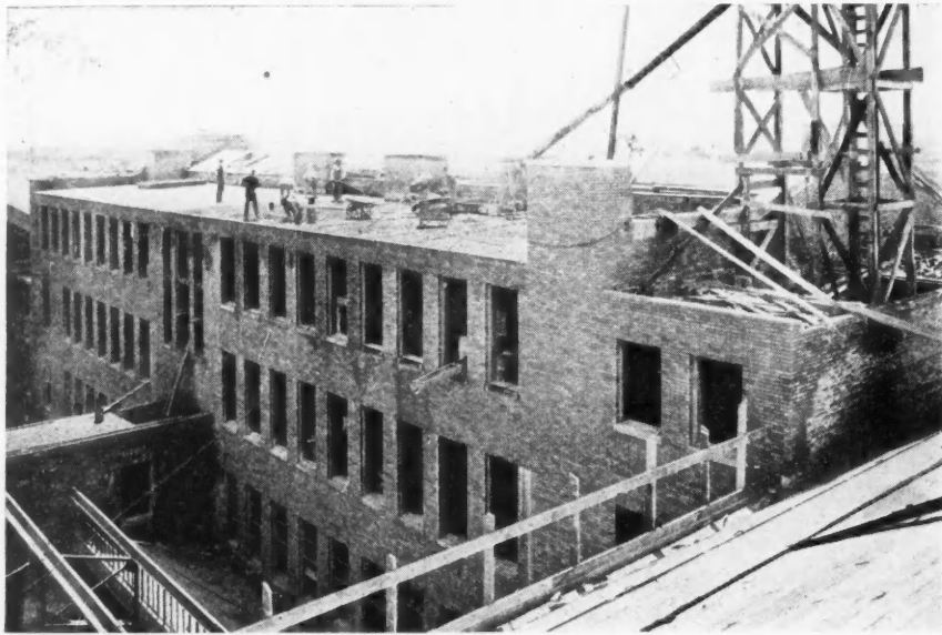
Laying the Roof, the Last Work on the Exterior of the J. Sterling Morton High School, Cicero, Ill. Concrete and mortar mixers and hoist were in natatorium in basement and material was elevated to different floors and piped by gravity to workmen.
