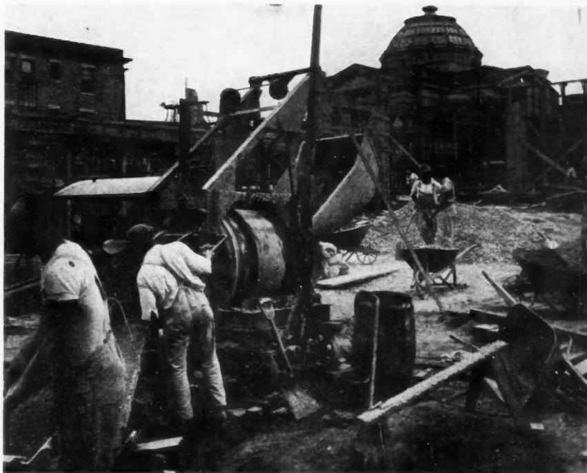
The J. R. Vansant Construction Company Found This Concrete Mixer Did a Large Part of the Work in Erecting the Worthman Office Building, at Kansas City.
