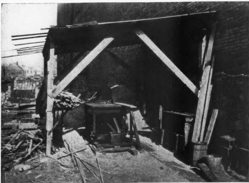
Taking the Saw Rig to the Building Job Is a Money and Time Saving Method. The Short Pieces of Timber Shown Here Will Be Used, as Each Can Be Quickly Cut to the Right Size for Blocking, Furring and Bridging. There Is No Waste Lumber on the Job Where a Saw Rig Is Used.
