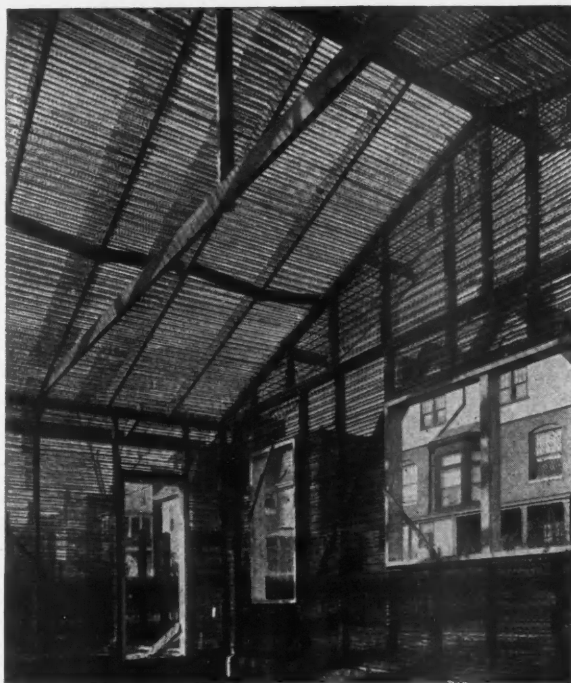
Interior View Before Plastering, Showing Outside Metal Lath Applied to the Studding and Wood Rafters.
