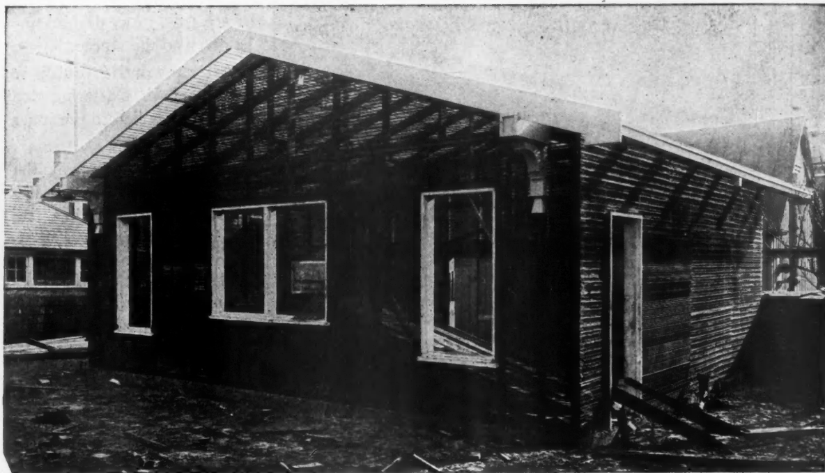
In Kansas City, Mo., Showing Ribbed Metal Lath on Wood Studding Ready for Stucco. Interior View of This Building Is Shown Above.
