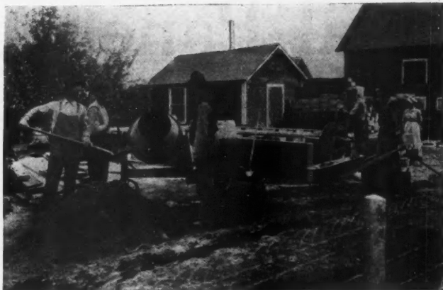
A Small Mixer Is Mighty Useful to the Country Contractor. Here Is L. Ebaugh and His Crew Laying the Floor After the Concrete Foundation of a Country Home, Near Clear Lake, Iowa, Had Been Put in.
