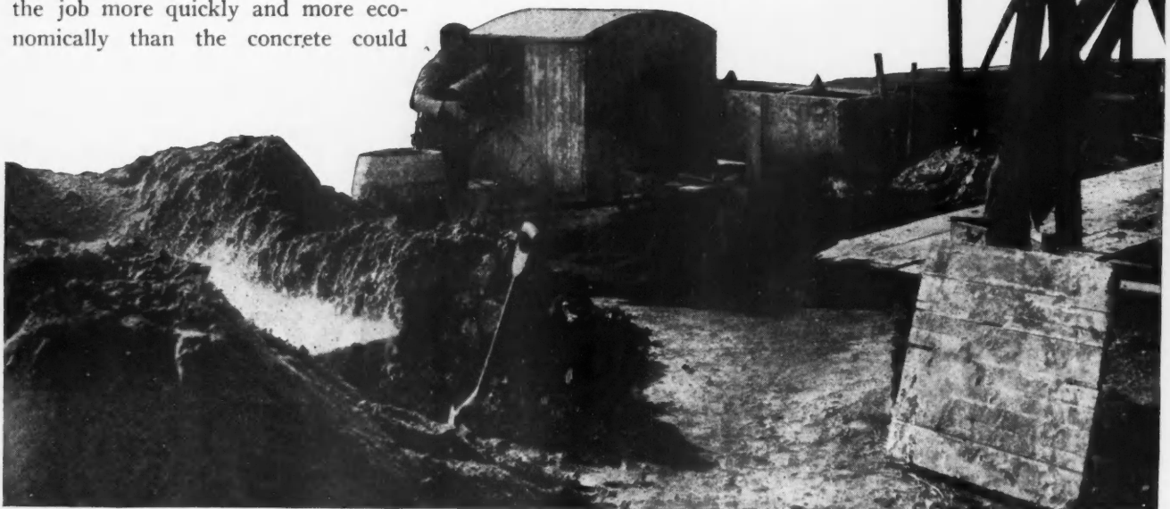
The Old Method of Mixing Mortar Has Been Superseded by the Power Mixer. It Does the Work Well and More Quickly Than It Can Be Done by Hand.
