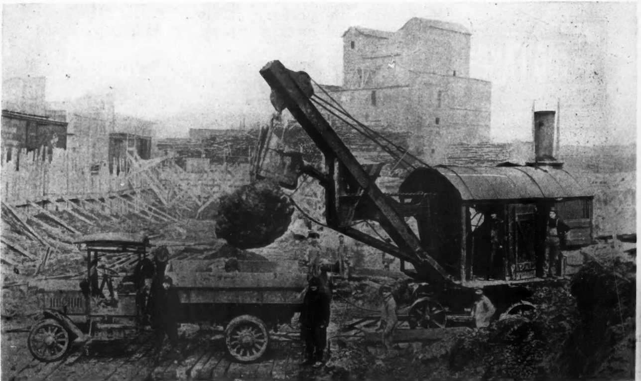
Tons of Dirt and Rock Are Taken from the Building Excavation by the Steam Shovel and Deposited in the Motor Truck. Here Is a "GMC" Truck Waiting for Its Load. Contractors Speed Up Their Work and Do It Economically with Such Motor Trucks.
