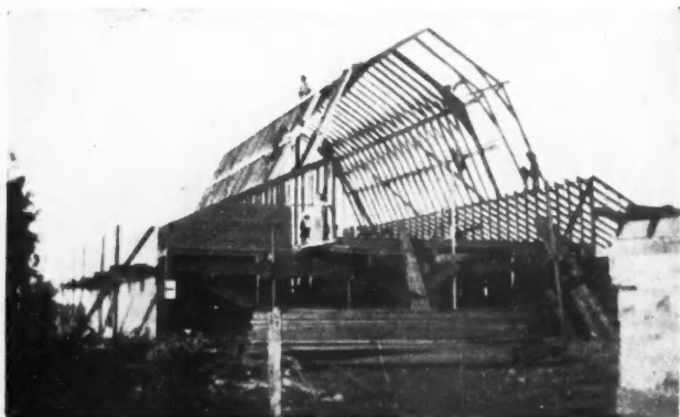
R. E. Vance and His Crew at Work on Gambrel Roof Barn.
