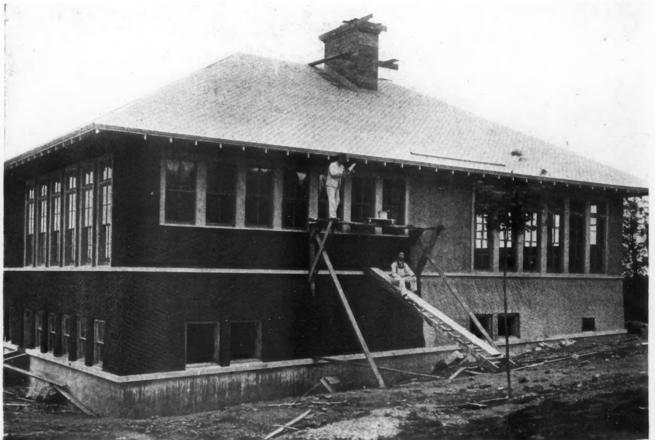
Reinforced Plastering Fabric on a Small School Building, Part of Which Has Been Covered by Stucco. The Backing Gives as the Stucco Is Forced Against It, the Plaster Sinking in and Keying on the Reinforcing Wires.
