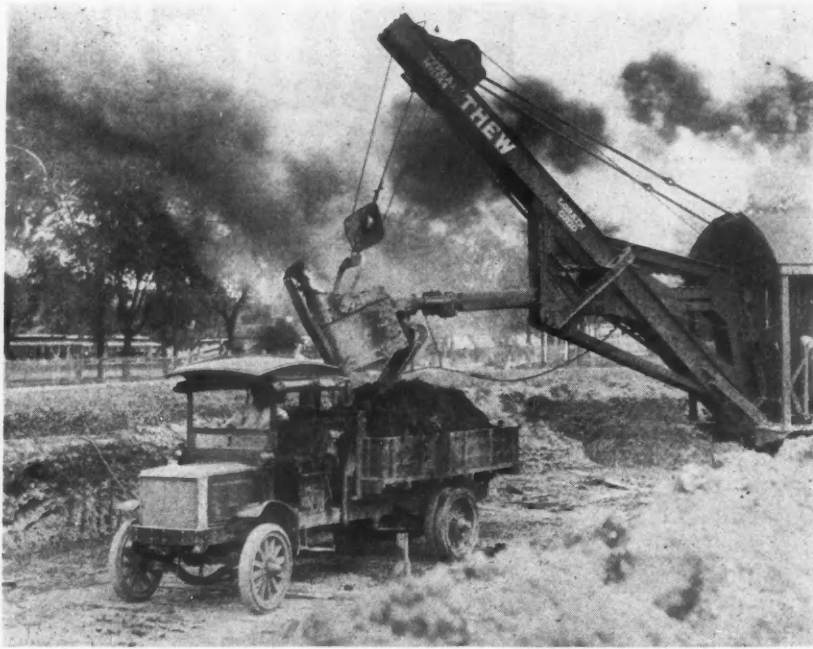
A "Federal" Truck Receiving Dirt from a Steam Shovel Excavating for a Big Building. Trucks Take Heavy Loads and Carry Them Up the Grade from the Excavation Easily.
