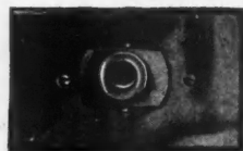
This receptacle requires a special plug restricting the use of devices to outlets similarly equipped. The ordinary push button switch plate is used to cover the outlet.
