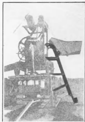
Mixer raised—track extended to charge mixer on same level with material piles.
