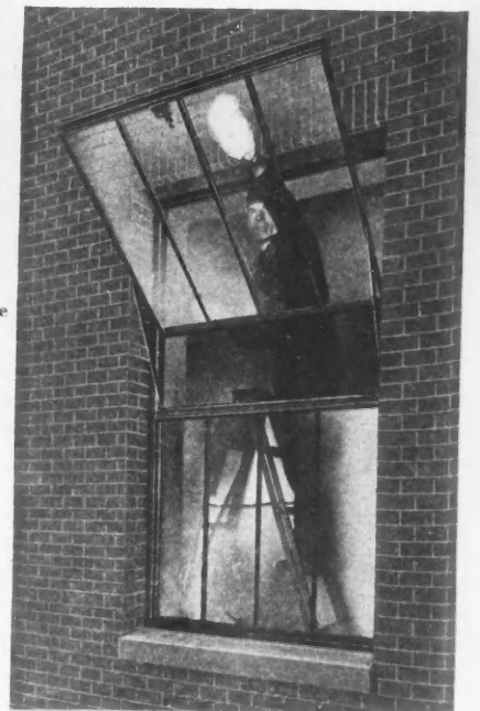
Balanced Ventilator Type. In This The Sash Are Balanced on Two Arms at the Jamb. They Can Be Reversed Easily for Washing From the Inside.
