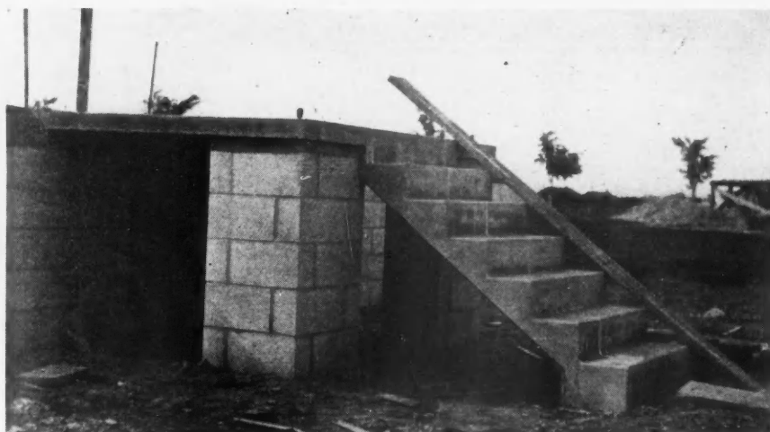
Fig. 4. Practical Flight of Concrete Steps for a Dwelling of Moderate Size. The Height of Riser is 7½ Inches and the Width of Tread is 10 Inches. Detail for These Steps and Attached Floor Slab is Shown in Fig. 5.
