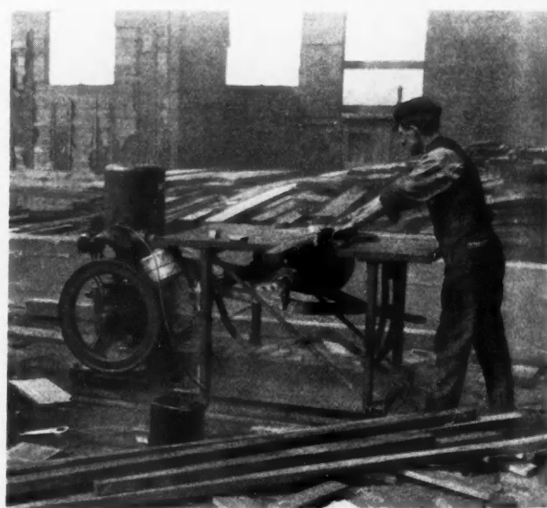
New Light Saw Rig Designed to Cut Labor Costs, Especially in Form Work for Concrete. It Has Many Attachments.
