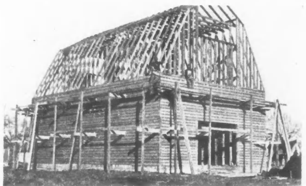
The Roof Framing of the Corncrib Completed, and Ready for Roof Boards and Shingling. Completed, the building has a 12-foot driveway 50 feet long, and inside elevator, 10-foot cribs, dump logs and deep pit, and electricity is used for power.
