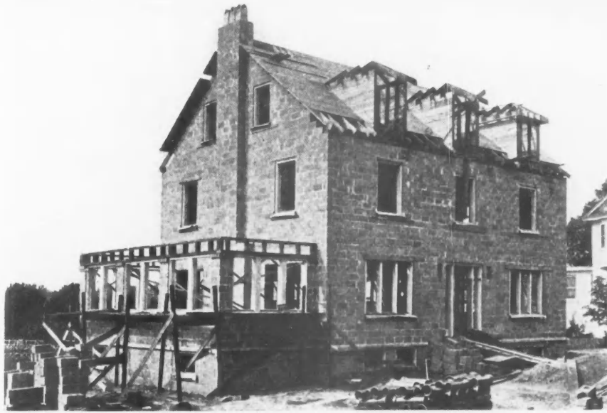
Typical of a Large Number of High Class Concrete Residences in Camden and Vicinity in Which Block from the Stock Pile of the Concrete Specialties Co. Are Used. This is a view showing block walls before cement stucco is applied.
