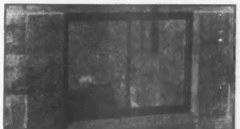
Grout in the jambs and sill, trowel the mortar flush, and the job is done. Total time—ten minutes.
