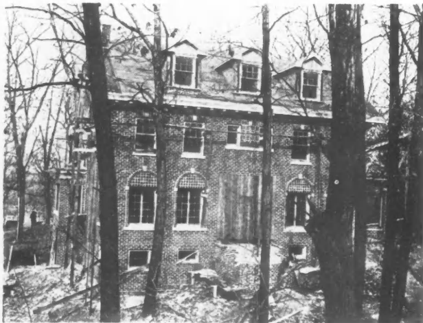
Residence at Oak Park, Ill., which the Atlas Educational Film Company is featuring in every detail of its construction, and which will form part of a film story which will be released in Own Your Own Home Shows Thruout the Country.
