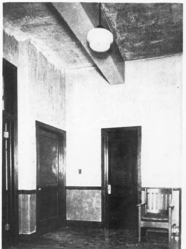
What Old Sizing Method Did to Walls: Alkali of Walls "Burned" Through, Ruining Paint.
