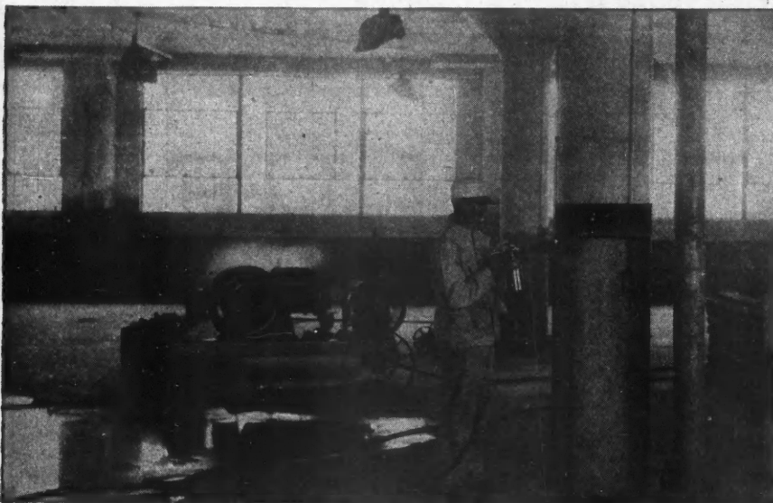
[Painting the dado—here the operator is using the DeVilbiss spray gun with Type I K N Pressure Feed Cup attached, which is advantageous on many kinds of work.]
