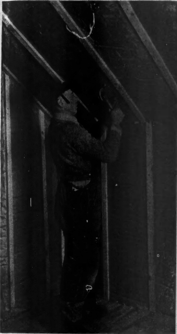
Every Insulated House That a Contractor Erects Is Another Turn of the Jack Under His Reputation for Good Houses.
