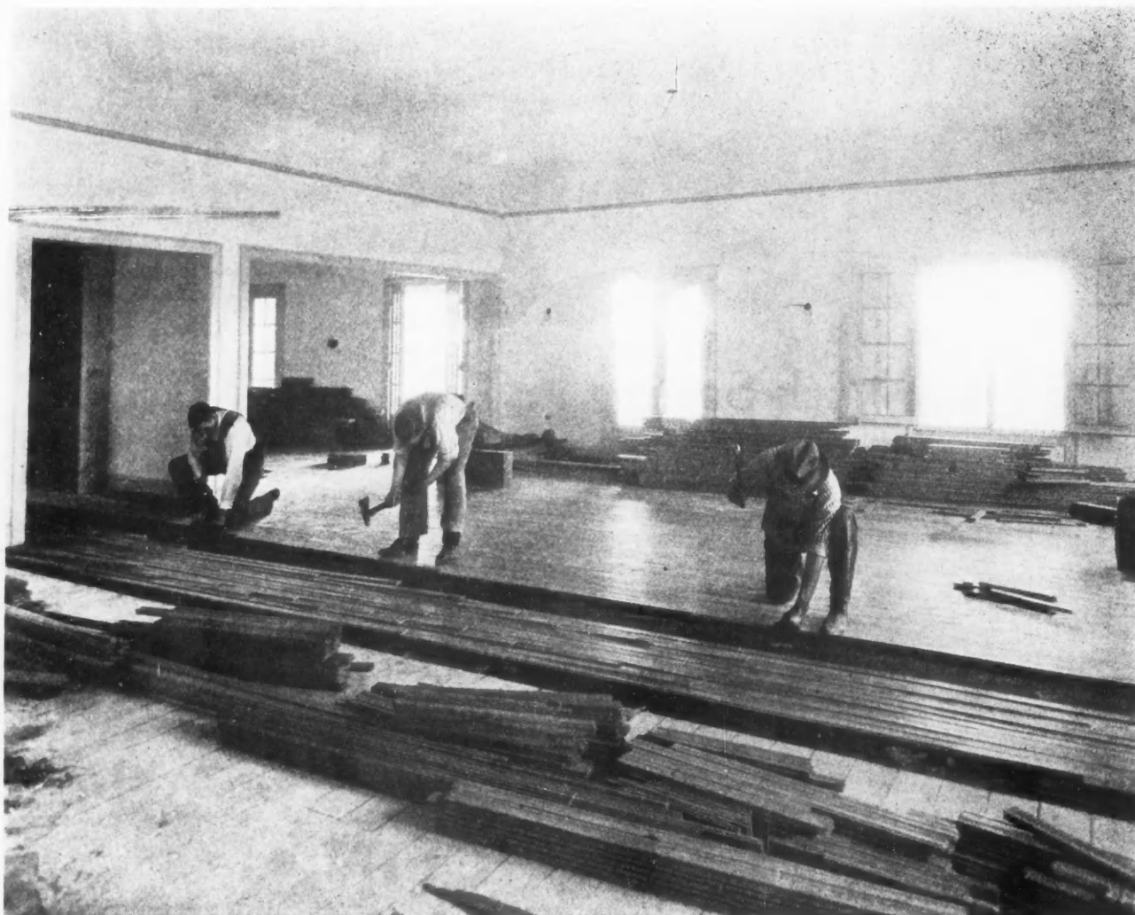
Workmen Laying the 13/16 Oak Flooring in the Community Recreation Association Club House, Evanston, Illinois. W. L. Claffey, author of this article, was chairman of the committee in charge of the construction of the club house, where his long experience in the building field proved valuable to the association he served.
