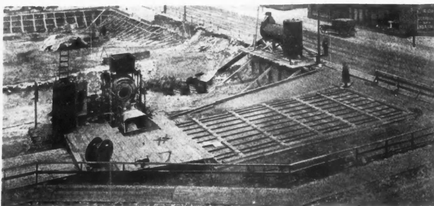
A Grillage of Steam Pipes for Heating Aggregate, as Installed by the Thompson-Starrett Company. As soon as the steam pipes have been covered with sand and gravel to a depth of three feet, steam is turned on in the pipe grillage and the aggregate kept at 70 degrees F. day and night.
