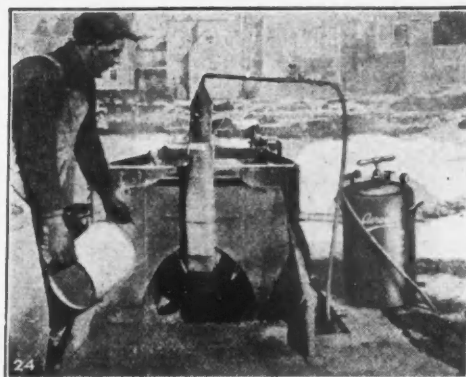
This device Throws a Kerosene Flame Within the Mixer Drum of a Concrete Mixer and Thoroughly Heats the Mix. It is said to produce hot concrete—from 70 to 90 degrees in winter weather. Further details will be furnished on request.
