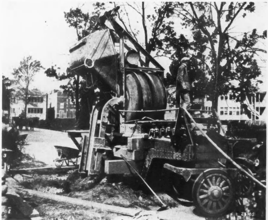
Mounting This Mixer on a Special Type of Trailer and Providing Special Hoisting Equipment Greatly Facilitate Pouring Concrete for Lamp Post Bases.
