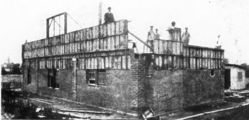
A Building of the Structural Gypsum in the Process of Construction. Note that the forms in which the material is poured are still in place at the top of the wall.
