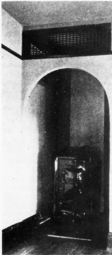
Special Hallway Location for Heating Plant Provided in Cellarless House Design. Note the openings left for free circulation of warm air at ceiling level.
