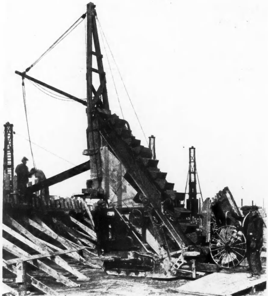
Using a Self Feeding Loader Instead of a Tower for Pouring Concrete.
