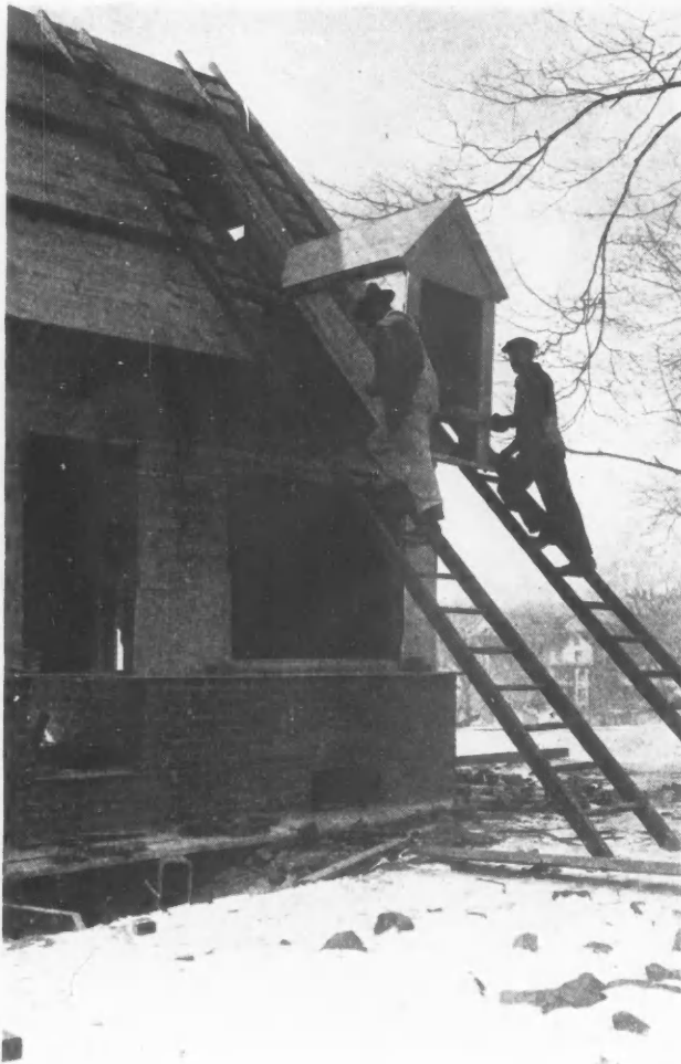
A Good Many Roof Dormers of Uniform Size and Design Were Required. They were all shop-built and quickly set in place on the roof.
