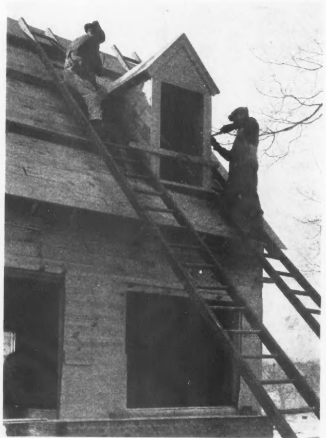
Each Dormer Weighed About 240 Pounds. They were easily handled. Why do work at a disadvantage on an awkward roof slope that can be more quickly and better done in the shop?
