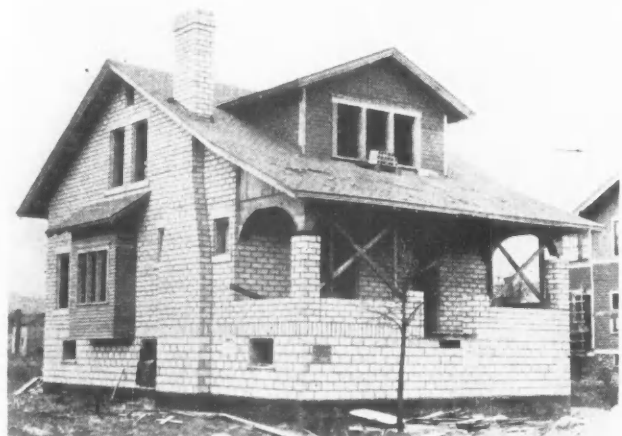
House of Concrete Tile in Course of Construction. A stucco finish coat may be applied over this if desired.
