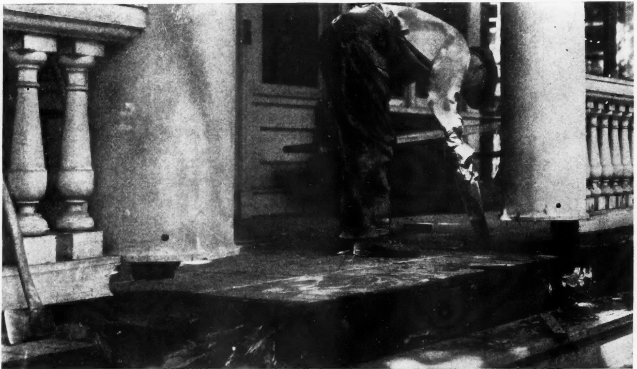
Lumber in Contact with the Earth Becomes Infected with Rot Fungi, Unless Protected. When steps and porch boards rot because of inadequate protection, the home owner is put to much unnecessary trouble and expense which could be avoided by the use of paint.
