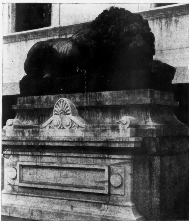
The Unsightly Stains Which Mar This Figure Could Have Been Prevented If a Metal Protective Paint Had Been Used on All the Metal Parts.
