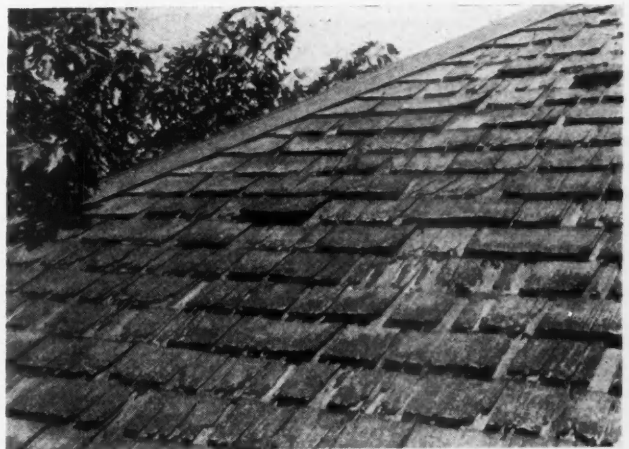
The Way of All Neglected Roofs. Paint would have kept off decay but now the owner must bear the cost of an entire new roof.
