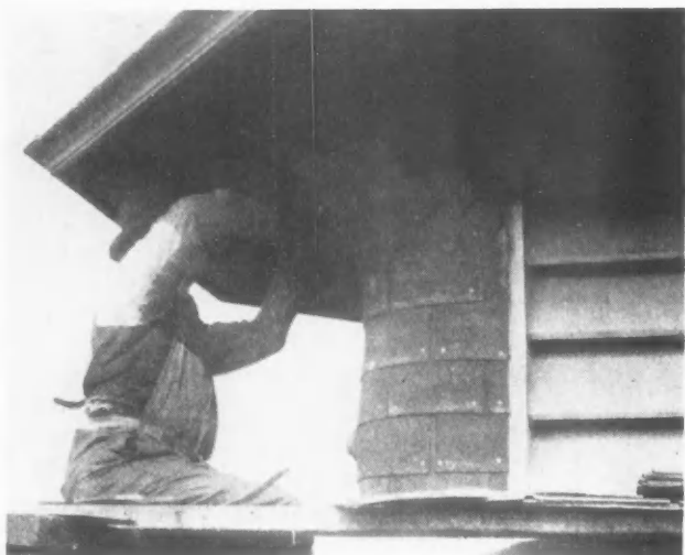
Applying Copper Coated Composition Shingles Which Bring a Copper Roofing Within the Means of the Average Home Builder.
