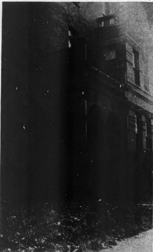
The Discoloration of Masonry Known as Efflorescence Disfigures Many Buildings But It May Be Avoided by Those Familiar with Its Causes.
