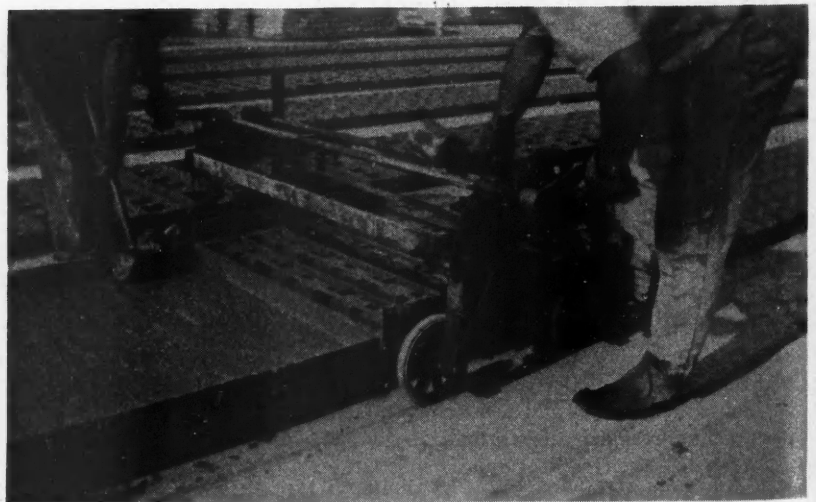
A Stripper, Which Lifts the Mold Without Disturbing the Freshly Cast Units, and a Mix of a Special Consistency, Make Possible a Remarkably Rapid and Economical Process.
