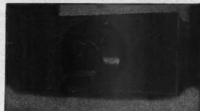
This shows fan in operation. Louvers close automatically when fan builds up positive pressure air circulation. Without the “automatic louvers” you could not have a successful “Forced Air” System.
