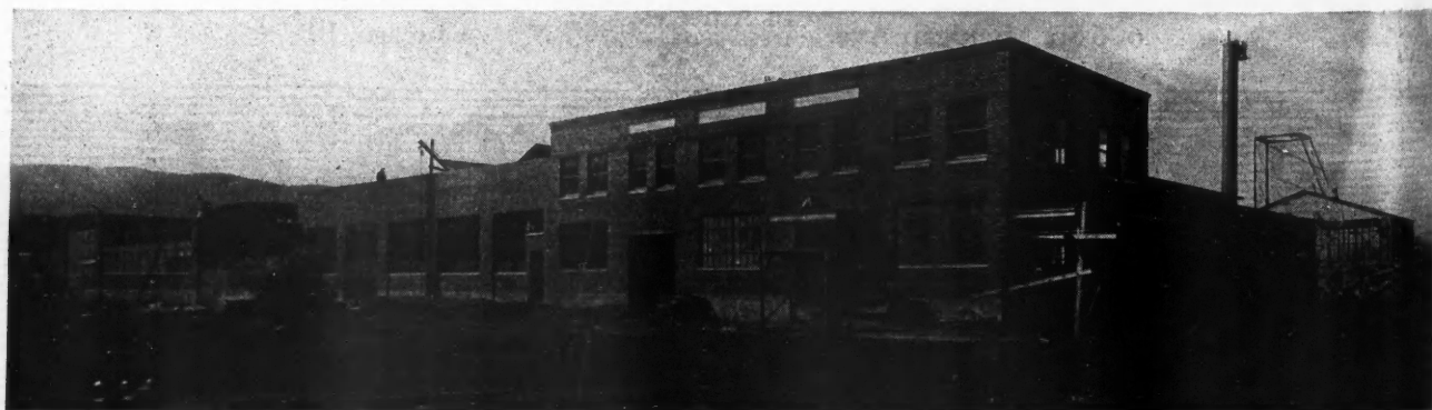
A Front View of the New Crooks-Dittmar Company Plant, with the Power House in the Background, as It Appeared During Construction. This has been called the most modern woodworking plant in the country.
