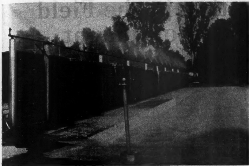
Twenty-Four Hours After Casting the Units Can Be Removed from the Casting Bed to the Stock Piles for Seasoning.
