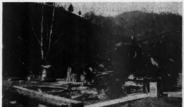
A Hoist-Compressor Combination for Steel Erection Where Permanent Installations Are Not Practical.
