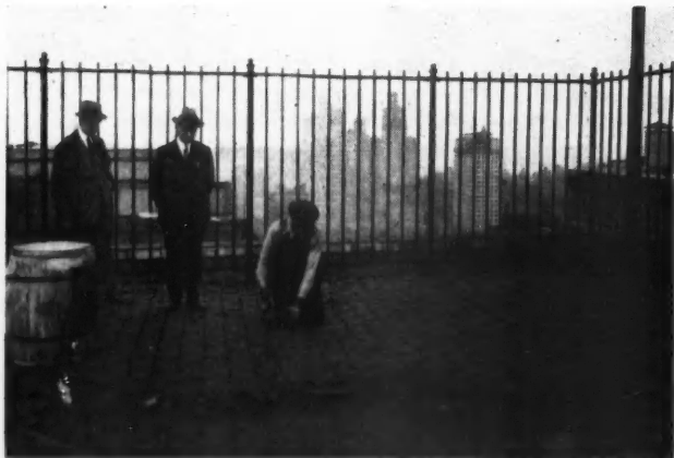
In Making a Permanent Repair of This Tile Roof the Workmen First Broke Out All the Original Setting Material That Had Become Hard and Brittle.
