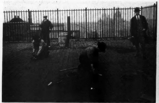
The Next Step Was To Caulk the Cracks Between the Tile With a New Asphalt Compound Which Is Quickly and Easily Applied.
