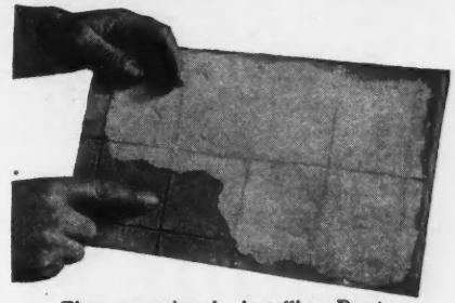
First operation in installing Porstelain Tile Walls. Foundation sheet covered with thin coat of Porstelain Cement.
