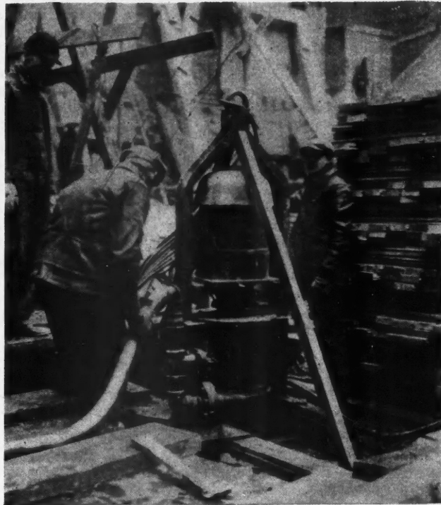
A Specially Designed Pump Widely Used in the Drainage of Caisson Holes Where "The Chicago Method" Is Used Features Reliability and Accessibility. Below: A more detailed view of the pump shown above.
