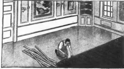
After breakfast—the room cleared and the carpenter ready to nail down the finished CROMAR Flooring.
