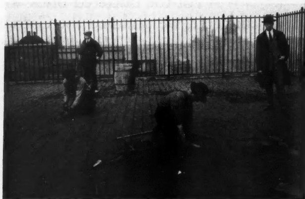
The Next Step Was To Caulk the Cracks Between the Tile With a New Asphalt Compound Which Is Quickly and Easily Applied.
