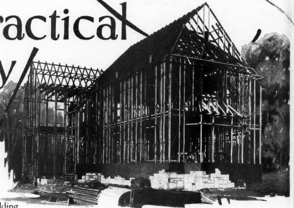
General view of typical steel frame for residence, erected in a fraction of the time necessary for old-type residence framing.
