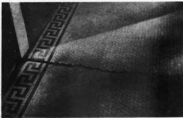
Fig. 2—Tile Surfaced Porch Floor, Showing a Large Crack in the Tile, Due to the Rotting Out of the Form Lumber Left in Position Beneath.
