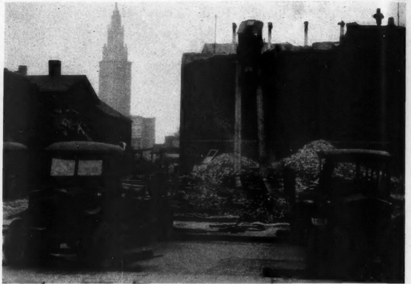
A Five-Ton Crane, Mounted on a Five-Ton Truck, Being Raised to the Fourth Floor of the Armour Building in Cleveland. A 1,500-pound skullcracker was swung from the end of the crane boom to demolish the building. In the foreground are two winch trucks pulling the crane up two 20 by 20-inch, 62-foot skids.
