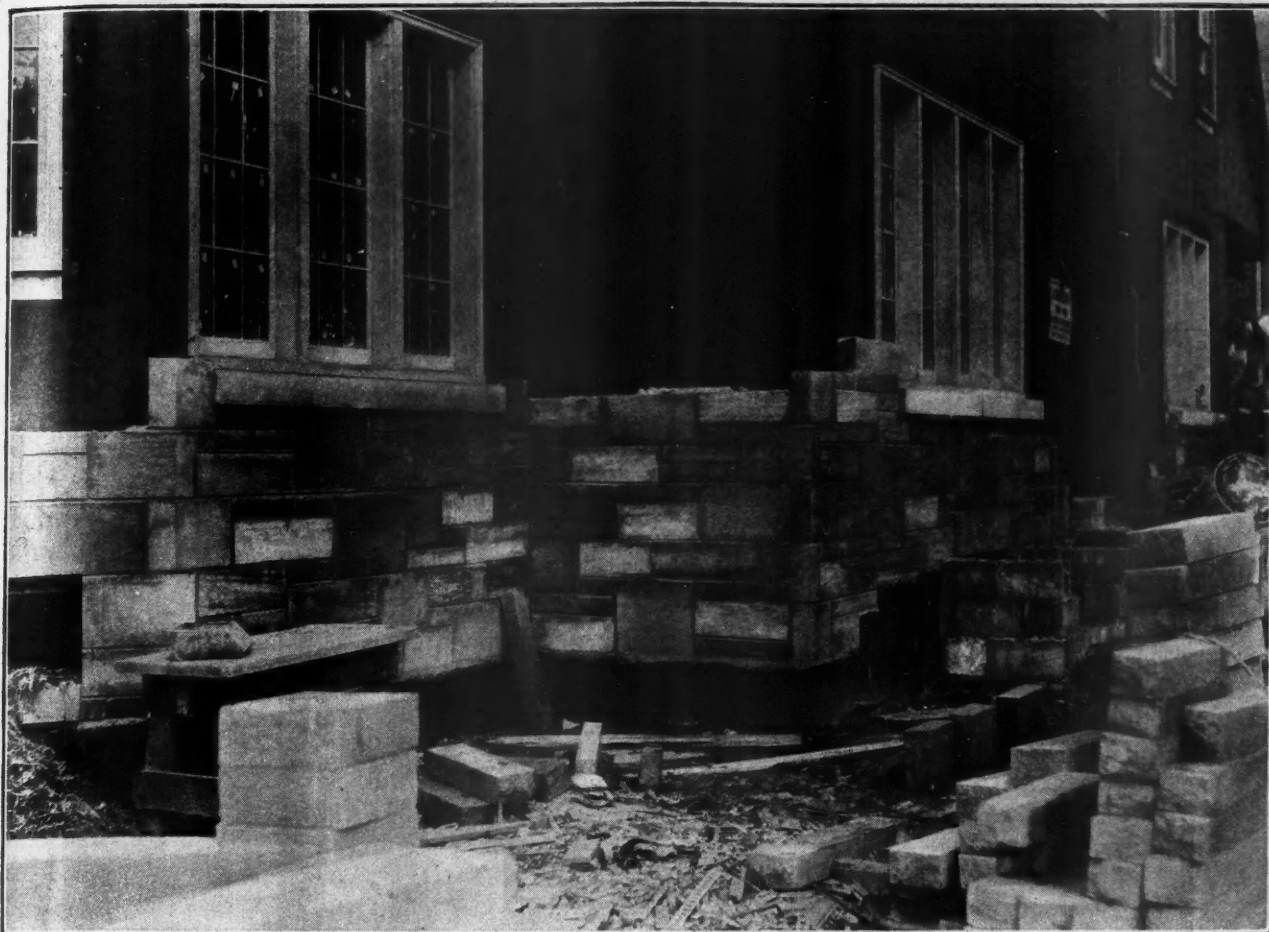
Laying up the stone in the Farley residence shown here. We co-operate with you on your first Indiana Limestone job so that you have no difficulty in learning how to use this beautiful stone.
