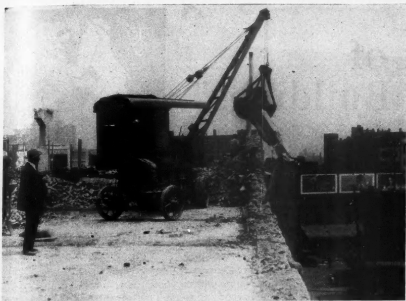
About 10 Per Cent, or Less, of the Time the Crane Used Its 1/2 Yard Clamshell Bucket to Clear Away Broken Parts That Fell on the Floor Instead of Over the Side of the Building.
