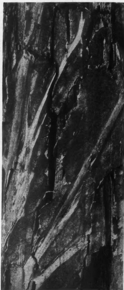
Fig. 11—Water-Conducting Strands on the Underside of the Pine Flooring, Laid Over Brick, Shown in Figure 3.
