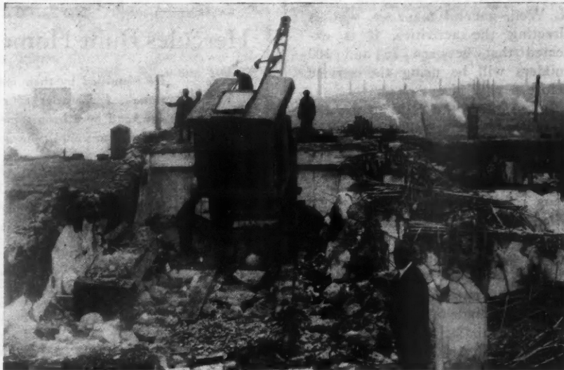
Here the Crane Is Being Lowered from One Floor to Another on Two 12 by 12-Inch, 20-Foot Timbers. One winch truck below is doing the lowering. Conrad Lurie, the contractor handling the job, is standing in the foreground.
