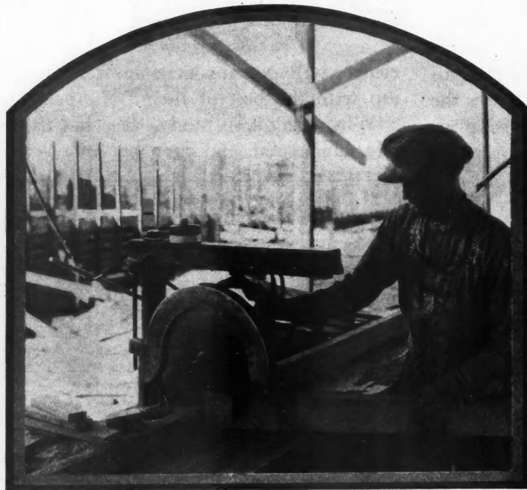
The Contractor Who Is Well Equipped with Modern, Labor-Saving Equipment Acquires a Prestige Second in Value Only to His Saving in Costs. Here a useful power saw is working its way.
