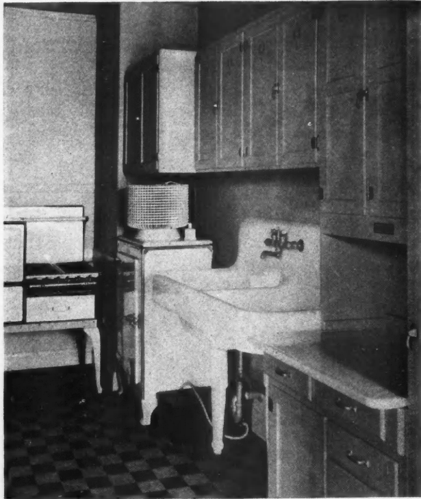
Each Apartment in the Building Is Equipped with All the Most Modern Conveniences, Including an Individual Electric Refrigerator Operating Independently.
