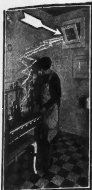
An ILGAIR Installation in an Oak Park, Illinois home. Note how the cooking odors, steam and fumes are removed.
