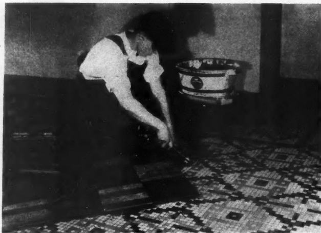
Laying Nine-Inch Treated Blocks in Mastic, Over an Expensive Mosaic Tile Floor in the Peabody Hotel, Memphis.
