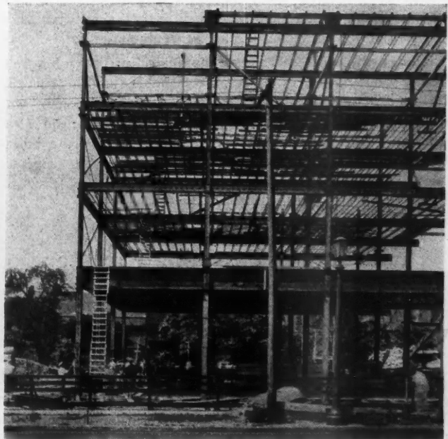
A Reduction in the Size of Columns from Floor to Floor Was Made Possible by the Use of Continuous Beam Design.
