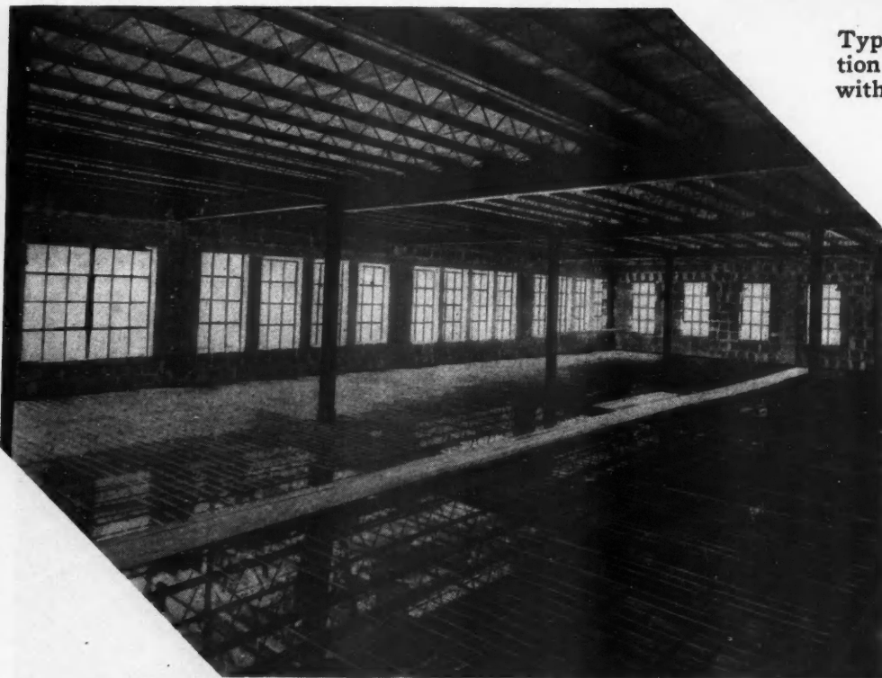
Using Open Web Joists, Several Floors Can Be Erected Without Waiting for Plumber's, Steamfitter's and Electrician's Installations and the Floors Can Be Poured Under Cover After the Roof Is Applied
