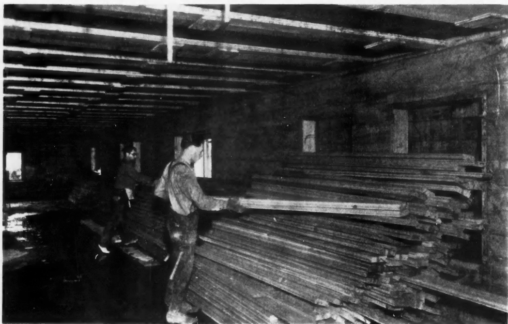
Step 2—When the concrete floors have set the 2 by 6 tongued and grooved shores are taken down and piled until needed for the partitions.
