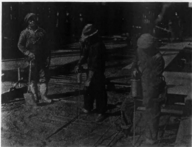
This Vibrator, Which Can Be Operated All Day by One Man, Without Fatigue, Is a Valuable Piece of Equipment in Producing High Grade Concrete.
