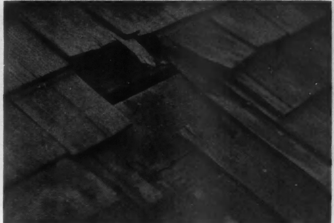
Rusty nails rot wood around them and shingles come out as they have on this roof.
