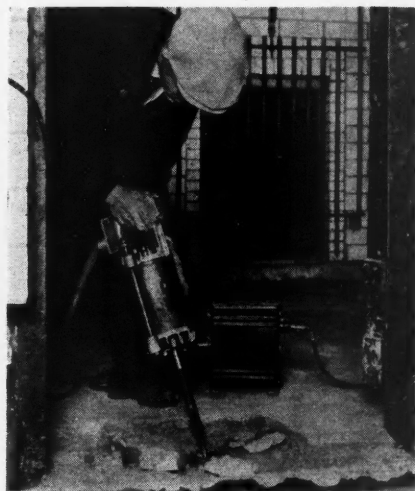
Chipping out concrete is a frequent modernizing job that is expensive without machine.
