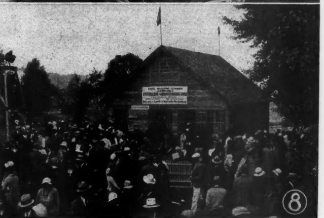
5. Noon—what 3 hours' work has accomplished; 6. At 3:00 P. M. the sheathing and siding were on; 7. At 3:30 at work on the roof; 8. The finished house.
