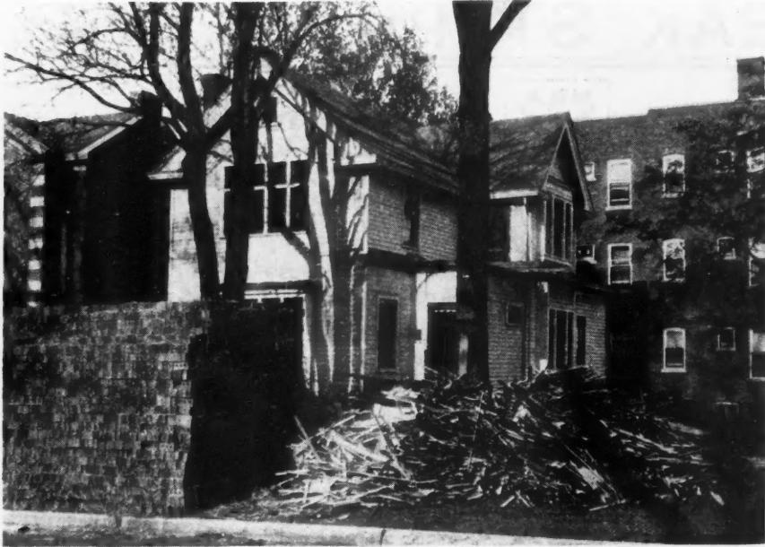
STEP 1: Tearing out old partitions, removing trim preparatory to remodeling. House of E. A. Lomas, Evanston, Ill., early this spring.
