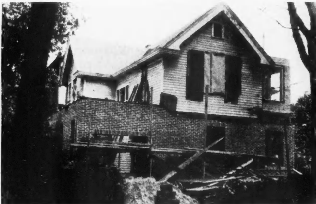
STEP 3: Building up rear of house and adding new garage. Small "den" was built over garage.
