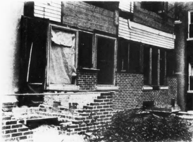
STEP 2: Laying up brick front and new entrance. New window frames were provided.
