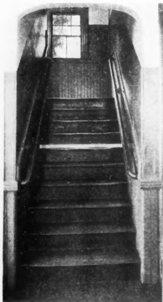
Worn stairs of a New England schoolhouse; "straight edge" shows how steps were worn.
