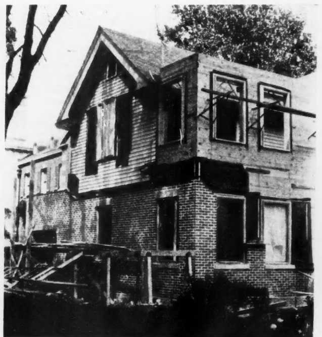
STEP 4: Adding to front of house by building on addition to make large upstairs bedroom.
