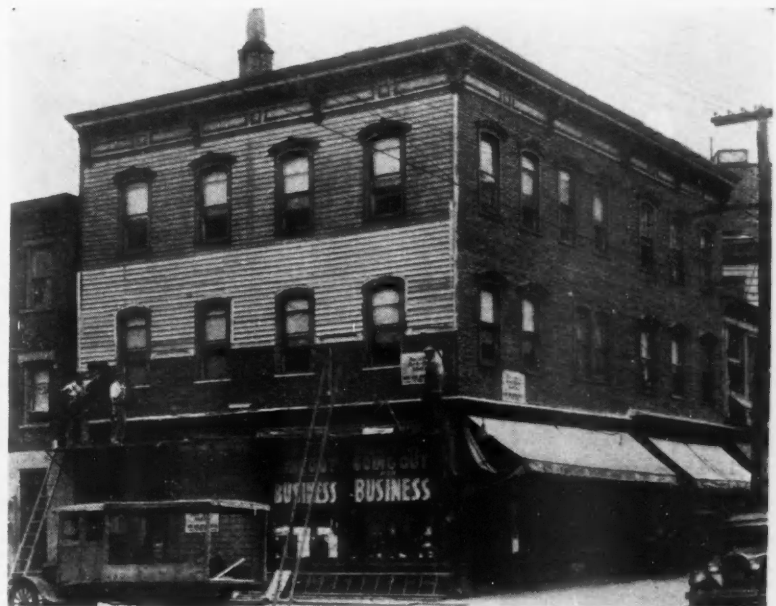
Business building in process of modernization in Newark, N. J. This job was done by The Globe Home Improvement Co. of Newark.
