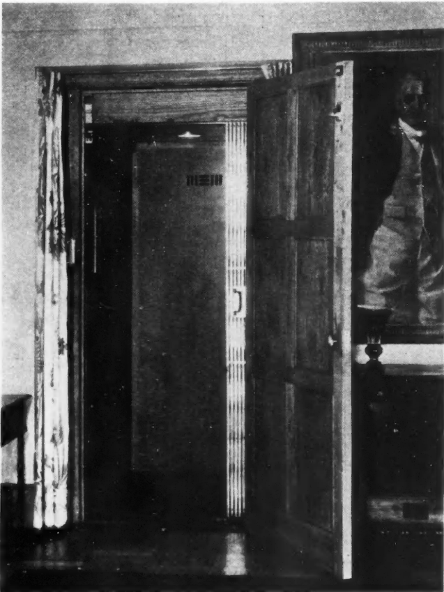
ILLUSTRATED ABOVE: Home of Ludington Patton, River Hills, Wis.; elevator shaft addition can be seen at the right end of house. At left: Interior view of the above home showing elevator car and door arrangement.
