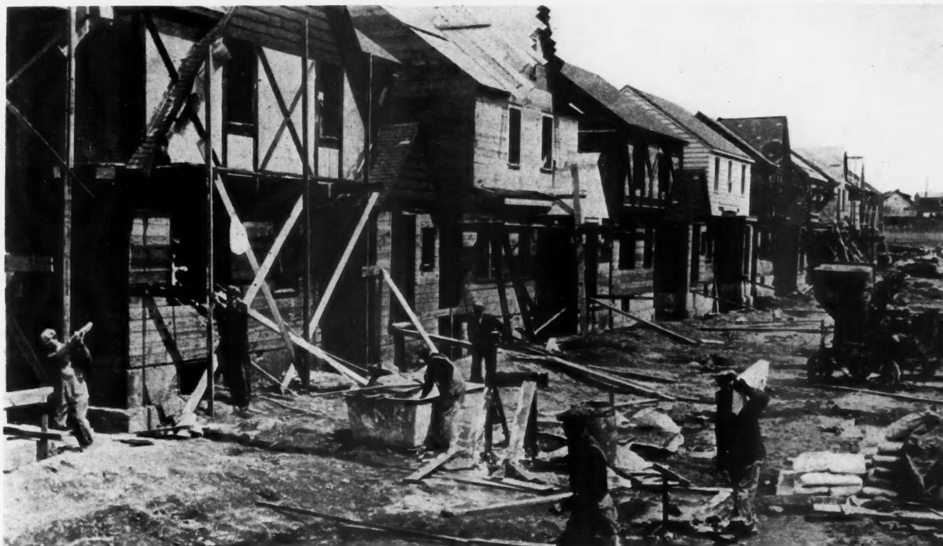
OPERATIVE BUILDERS are hard at work in the New York area supplying the pent-up demand for modest priced homes. Here is a scene at 169th Street and 25th Avenue (Flushing) where Bob Rose Developments, Inc., operative builders, have a large group of homes under construction. More than 250 are planned to be built this year.
