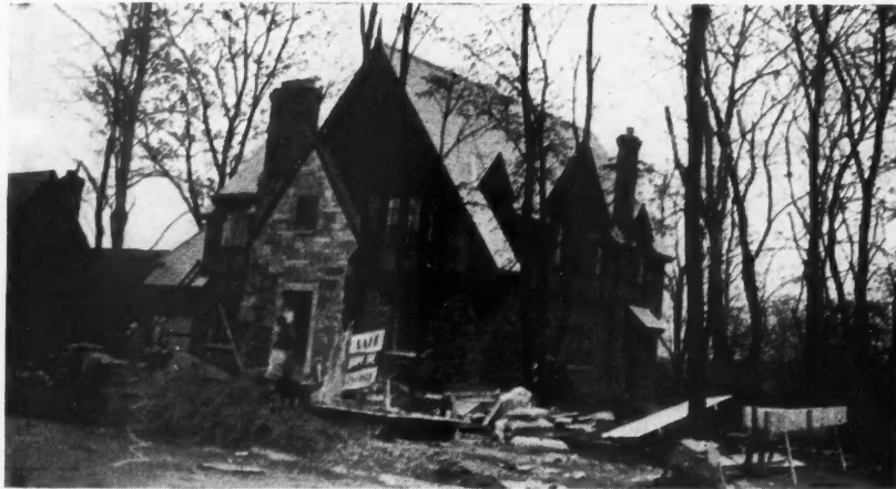
HOUSE under construction in Hyde Park section of Cincinnati photographed by American Builder on May 1; Herb Cassinelli, Builder; L. J. Marioni, Architect; Kopf & Kopf, sales agents. Price $21,000.
