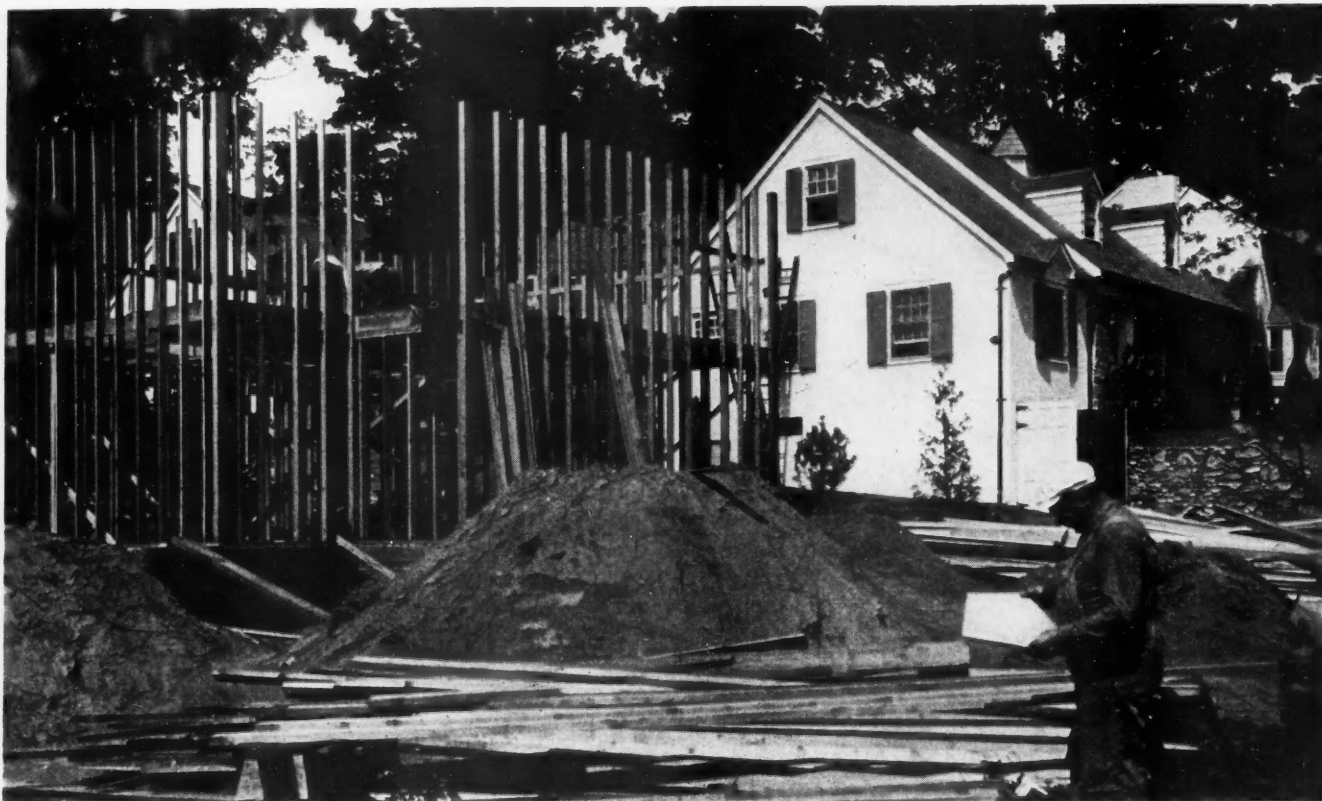
THE CONSTRUCTION CREW is working overtime at Strathmore-at-Manhasset to take care of quality home seekers
