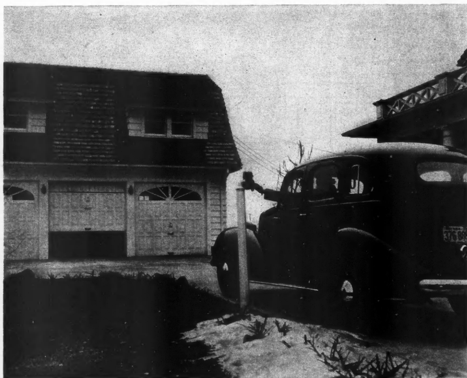
ABOVE is good example of distant control electric door opening; each of these three doors operated from one key switch post. Doors are "Overhead Doors" from the Overhead Door Corp. Charles H. Houck, architect, Muncie, Ind.
