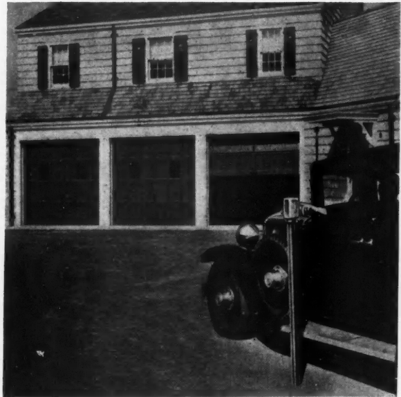
ELECTRIC operator controlling roll-up doors.
