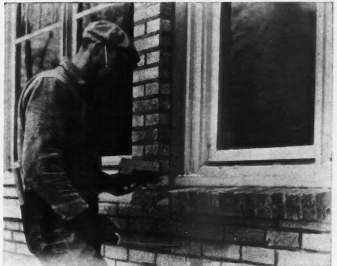
ABOVE: Workman laying corner brick for window sill. BELOW: Two-inch veneering tied to old clapboard wall with air space.
