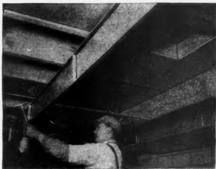
Even the trunks are standardized in the fully pre-fabricated Tempered-Aire duct system
