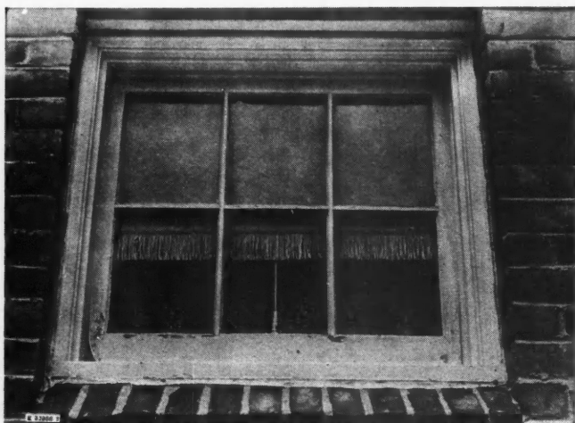
FAILURE of paint on the exterior of sash caused by condensation of moisture on the inside. A little bluestain shows through faintly in the photograph but in general the bluestain was most prominent on the inside surfaces. There was no condensation on this window when inspected.
