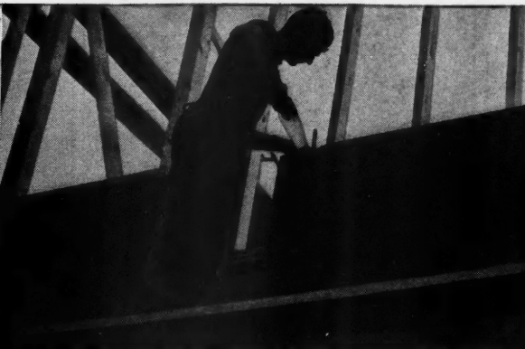
4 Cut-outs for windows and angles can be made on the scaffold instead of measuring and cutting on the ground.
