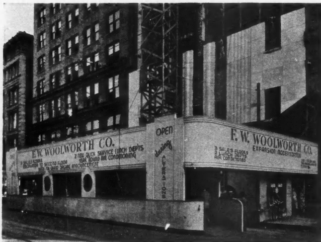
A TEMPORARY front which serves as an attractive advertisement during remodeling is shown here. The Douglas Fir Plywood is of the "EXTERIOR" grade, which is strictly waterproof, and is to be preferred where conditions of extreme humidity apply, or where extensive reuse is contemplated.
