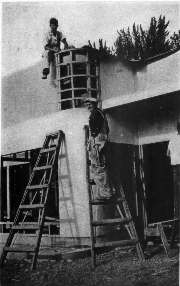
LATHS were used as reinforcing strips under the \frac{1}{8} " Exterior plywood panel on the rounded corners of the J. E. Windel streamlined grocery in Portland, Oregon. They also make a flush joint possible with the \frac{3}{8} " exterior grade used on the sides.
