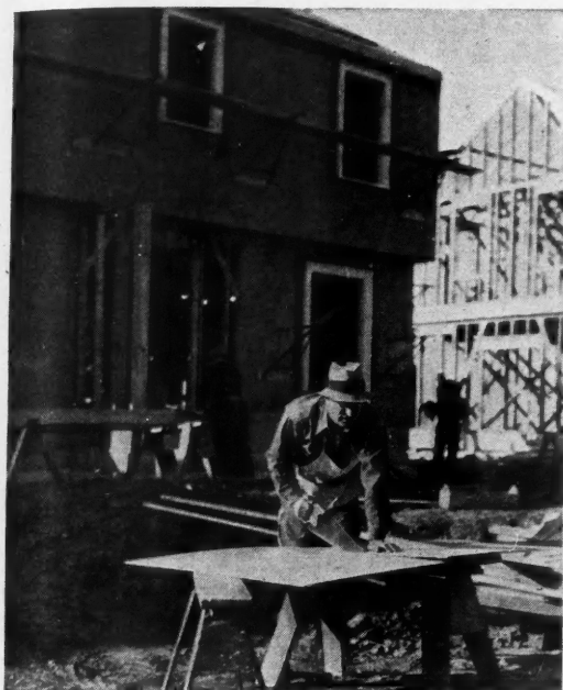
SPEED IN CUTTING and applying exterior plywood sheathing reduce time for enclosing house.
