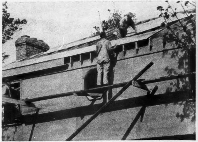
HERE the 5/16" PLYSCORD is laid as roof sheathing. On some jobs 3/8" may be used if rafter spacing and snow load make this advisable. Nailing strips are placed over the tight Plywood roof on this job and when the shingles are applied the extra air space will add still more to the warmth and insulation value of the roof
