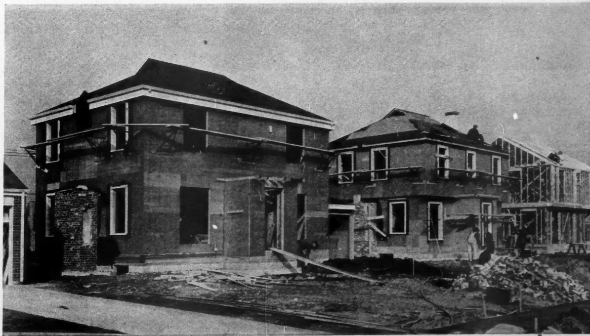
FAITH IN FUTURE is shown by Patrick Dwyer who started 15 new homes this fall because he believes good business is ahead. He uses 5/16" "Plyscord" sheathing for walls and roofs.
