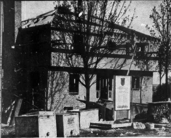
BRICK veneer was applied over PLYSCORD on the first floor. The rigid plywood under the veneer provides a warm and airtight undercoat for the house, and is a splendid nailing base for brick ties.
