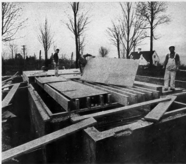
ABOVE: PLYSCORD sheathing now being laid for the sub-floor. Builders report time savings with this construction as high as 60% compared with laying a diagonal shi lap sub-floor. TOP PHOTO: Fitting \frac{5}{16} " PLYSCORD sheathing around an opening, emphasizing the minimum of cutting necessary, with plywood.
