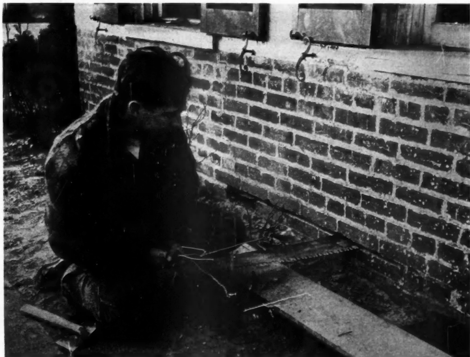
RIGHT: With a cross-cut saw short sections of mortar are readily removed; a second workman is inside on the other end of saw. Strips of sheet copper and asphalt roofing are inserted as the job progresses around the building to give a moisture barrier.
