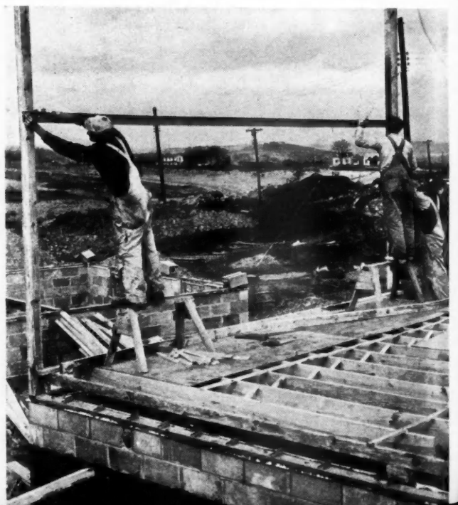
FIG. X—FIRST STEP IN FRAMING is erection of 4 x 4 corner posts into which steel ribbon with stud spacers is notched and nailed. Steel ribbon and sill act as templates, insuring exact dimensions so that precut lumber and prefabricated steel units will fit in place exactly.
