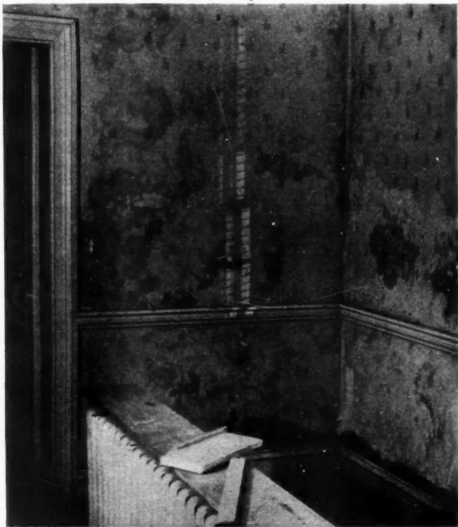
ABOVE: Interior of old house with solid brick walls laid in lime mortar showing damage due to water drawn from foundation by capillary action.
