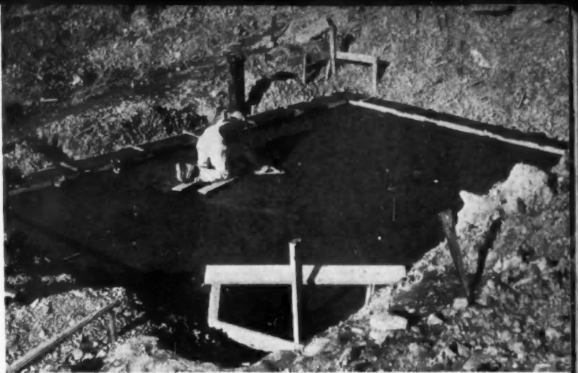
FIG. III—ONE PIECE FLOOR AND FOUNDATION —The monolithic concrete floor and footing with a 3½-in. raised edge are poured in one operation, thus eliminating a second return of the concrete crew. Plumbing and sewage pipes have to be laid before pouring is done.
