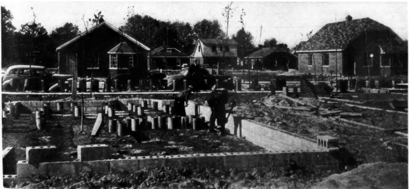
FOUNDATION construction of basementless homes at Villa Shores. Concrete floor slab poured on heavy metal lath rests on cement tile posts placed on about 3-foot centers.
