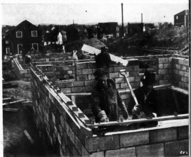
FIG. IV—HANDY GRIP, LIGHTWEIGHT TERRA COTTA TILES are laid up rapidly and a metal termite shield applied. Steel sill with welded stud spacer is then bolted to foundation in a bed of mortar.
