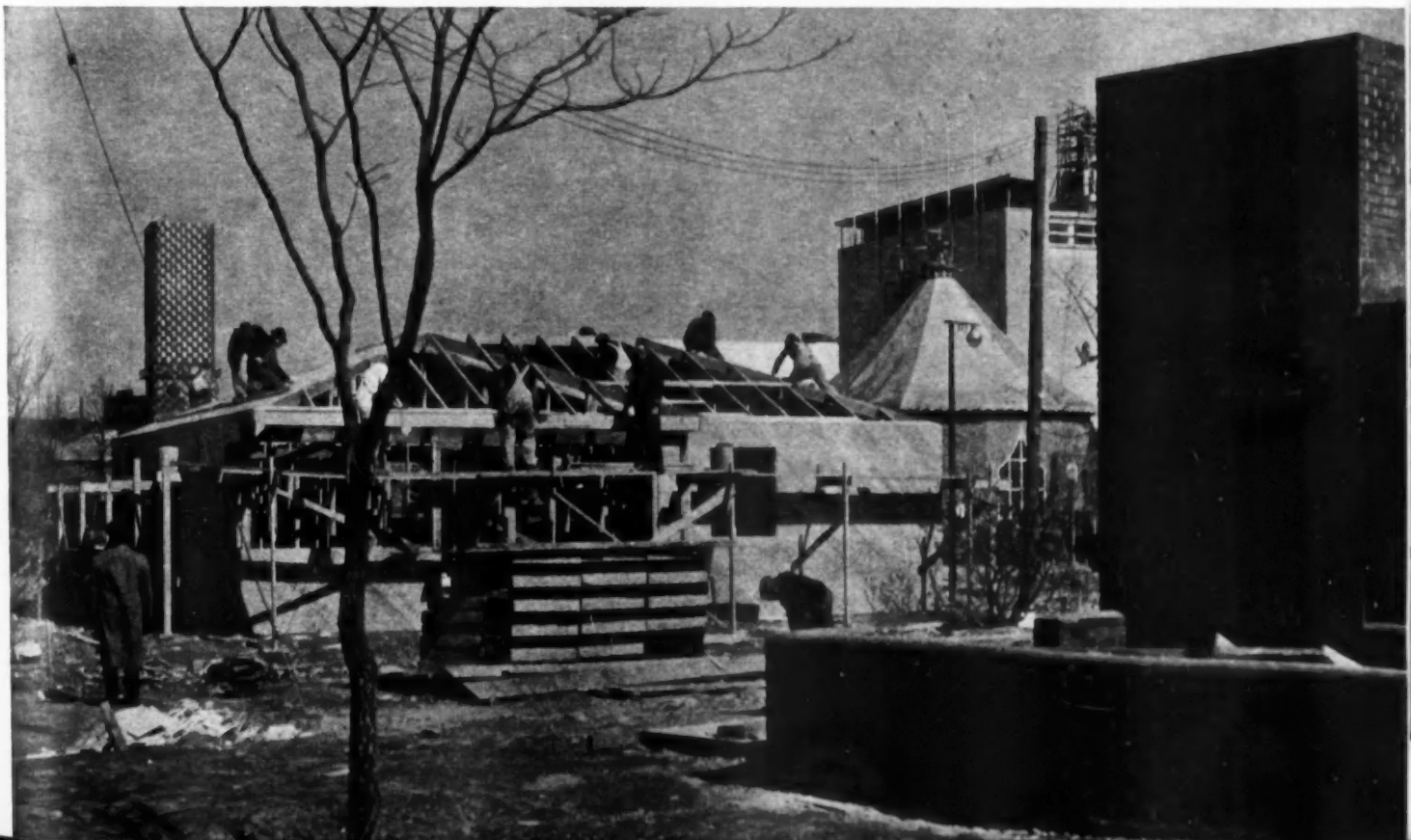
A BUSTLING SCENE OF ACTIVITY: In foreground is the low-cost lumber home sponsored by National Small Homes Bureau.
