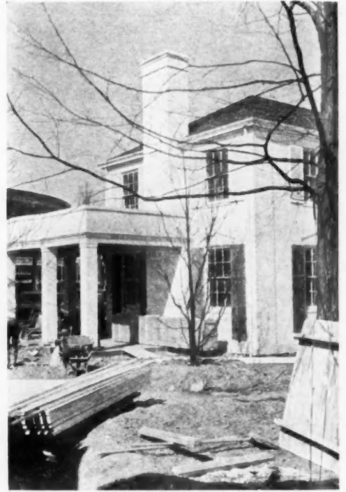
THE ALL-ELECTRIC HOME in fresh modern Georgian style brings the latest in equipment features.
