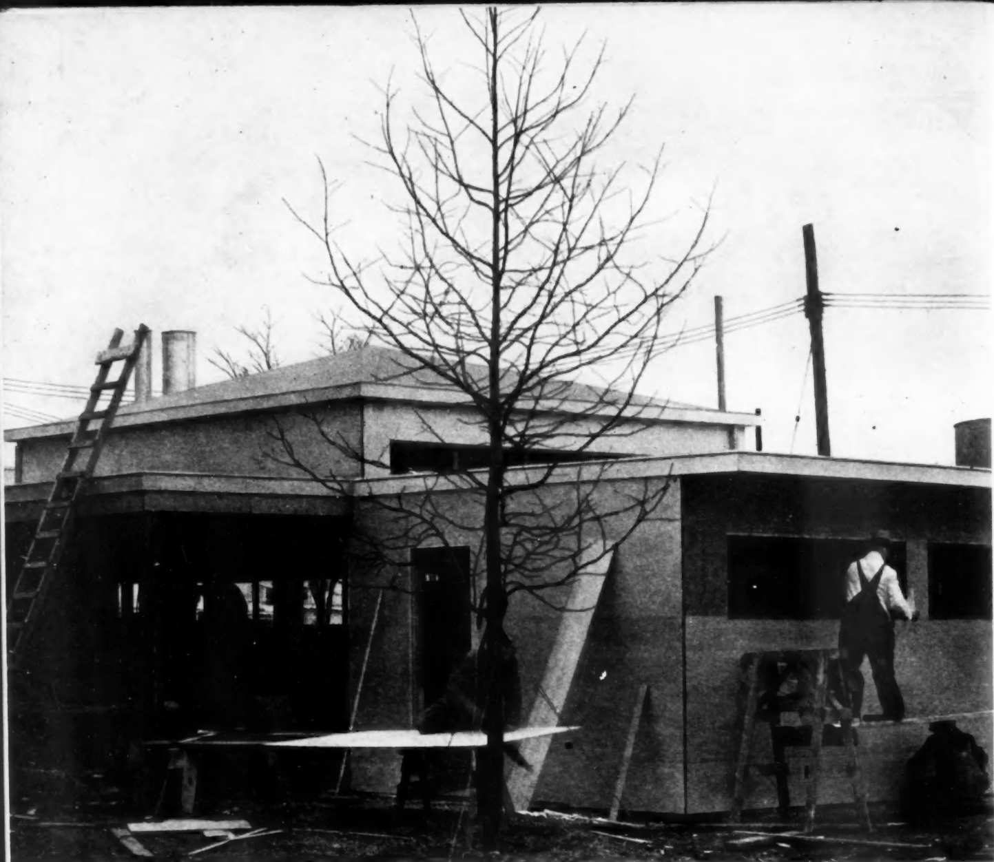
PROGRESSIVE prefabrication—scientific advance—new products—new "high value" for low cost—in Douglas Fir Plywood house at the Fair.
