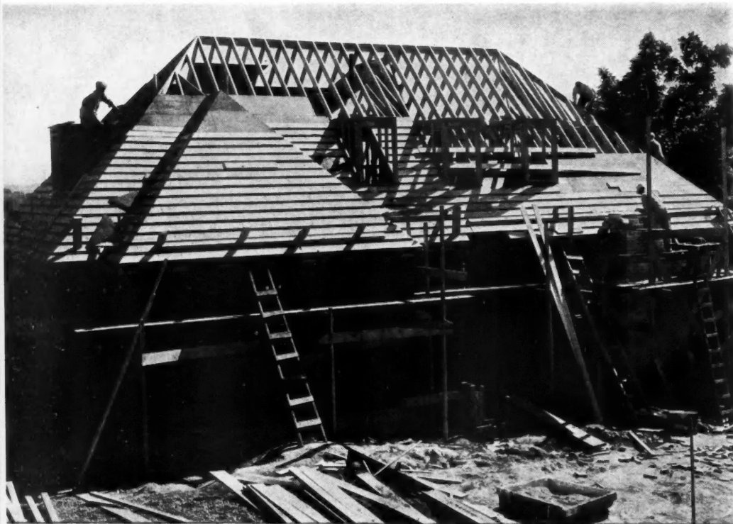
THIS construction view shows how roofers were laid over insulation board to take the red cedar shingles. Fir-Tex board was also used under T & G siding and as plaster base.
