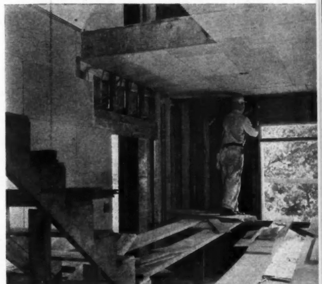
THE McCready home was sealed inside and out with insulation board for sheathing and plaster base, the latter applied as shown in the above view. The home has an air conditioning system.
