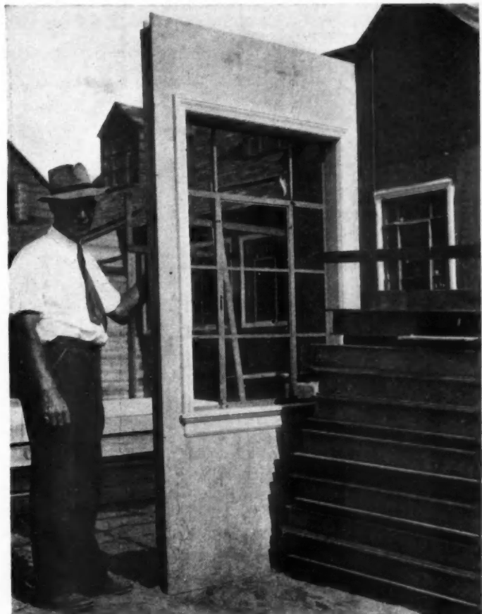
BILL WHYTE, JR., supports typical 4 x 8 plywood wall panel with window installed, complete with inside trim. Note how edge of panel projects to overlap next section.
