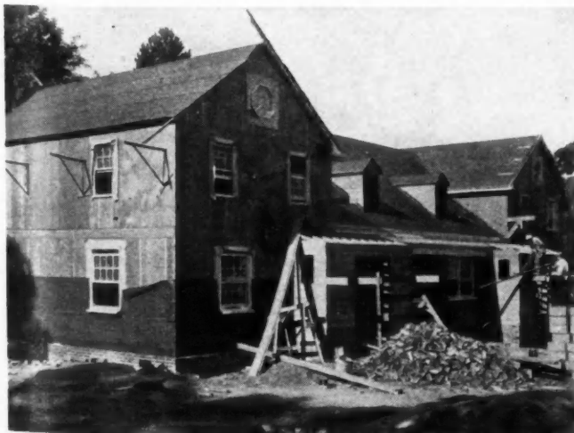
8—COMPLETED cottage apartment before addition of brick exterior. (Plans were shown in February '41 American Builder.)
