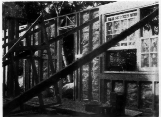
6—INTERIOR VIEW of panels shows bracing method, mineral wool insulation as installed at shop.
