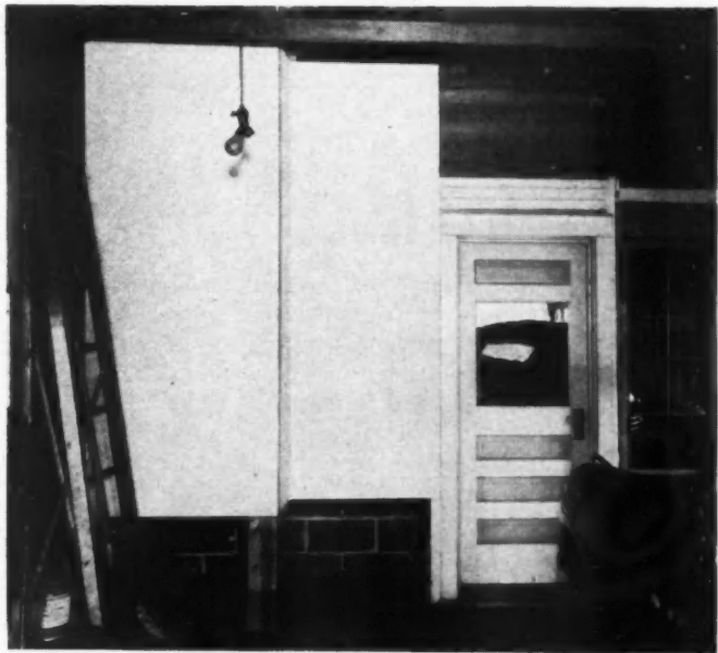
PHOTO above shows carpenter in new bathroom working on linen closet alongside of shower. Photo below shows garage with shower stall and linen closet projecting.
