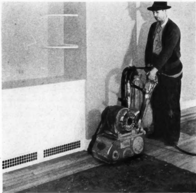
OLD OAK FLOOR in the living-dining room is being sanded. This room is covered with carpet, not nailed down, and this necessitated sanding and refinishing about one foot of the floor space around the walls. A power sander did this work effectively.
