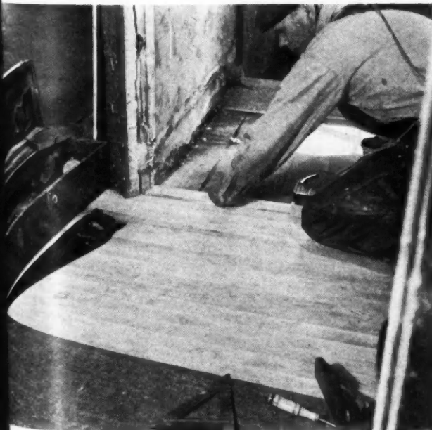
NEW MAPLE FLOORING in the hall; old flooring removed was used to patch other floors where registers occurred.
