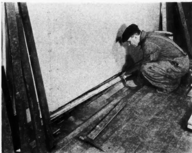
SUCCESSFUL PATCHING of the old floors throughout the house was accomplished speedily and easily. On the first floor the holes left from former hot air registers were patched with similar old flooring taken from the front hallway.
