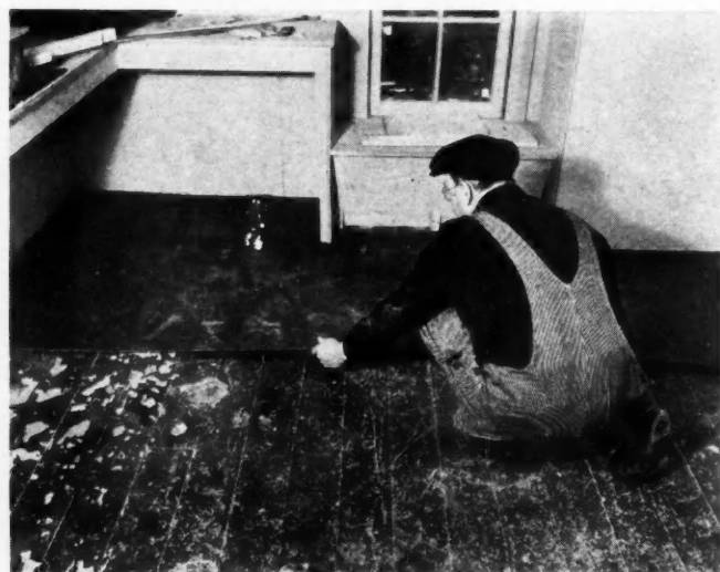
Here we see \frac{1}{8} " Hardboard being laid on the soft pine sub-floor of the bathroom, as a smooth base for the medium grade, marbled inlaid linoleum floor. Hardboard is also used as a base for the linoleum in the kitchen and powder room.
