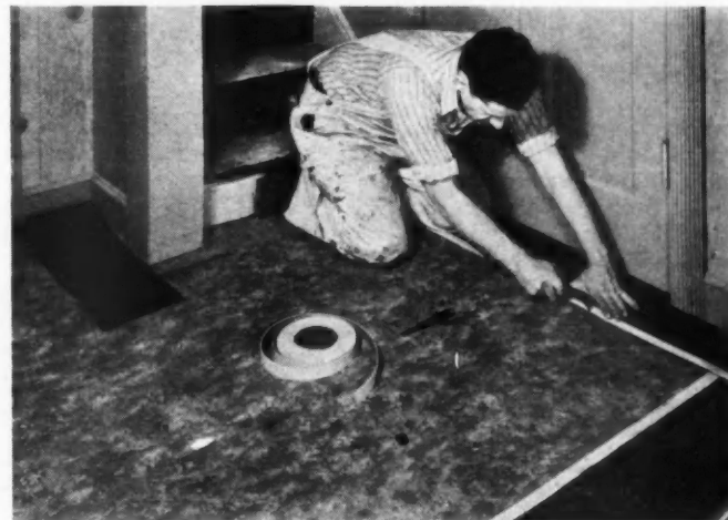
HERE, a workman is completing a skillful and ingenious flooring job. The floor level was corrected to provide for the new linoleum finish, which is a blue marbled pattern with a 6" black border strip, separated from the field by a band of white.
