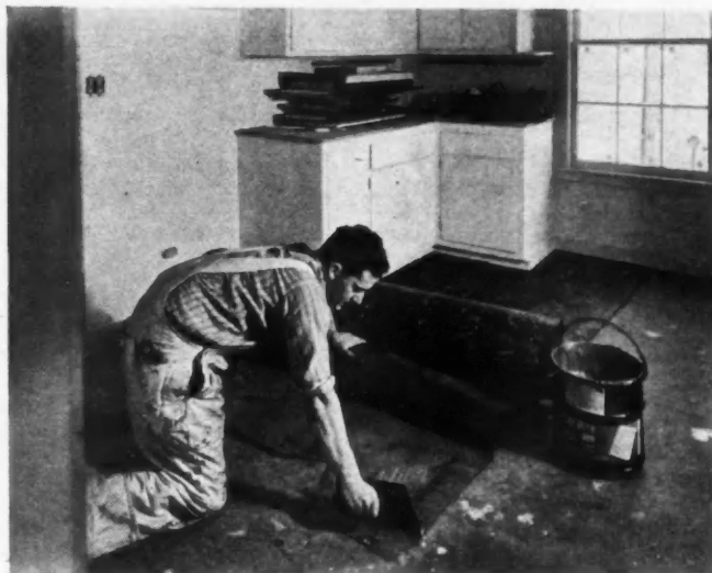
CAREFUL preparation was made for the new marbled linoleum in the kitchen. Here a workman is spreading Lay Rite linoleum cement over the USG Hardboard, which had already been applied to insure a flush base.
