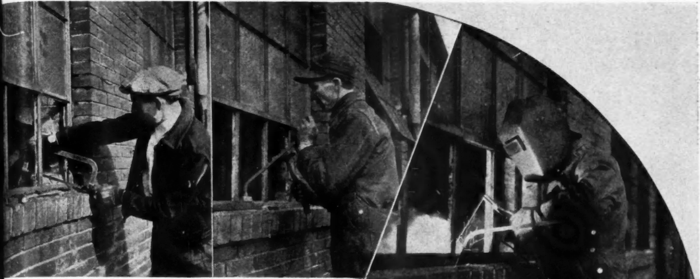
RUSTED bottom sill member is hack-sawed out, new piece welded in; sash are then reglazed and caulked.
