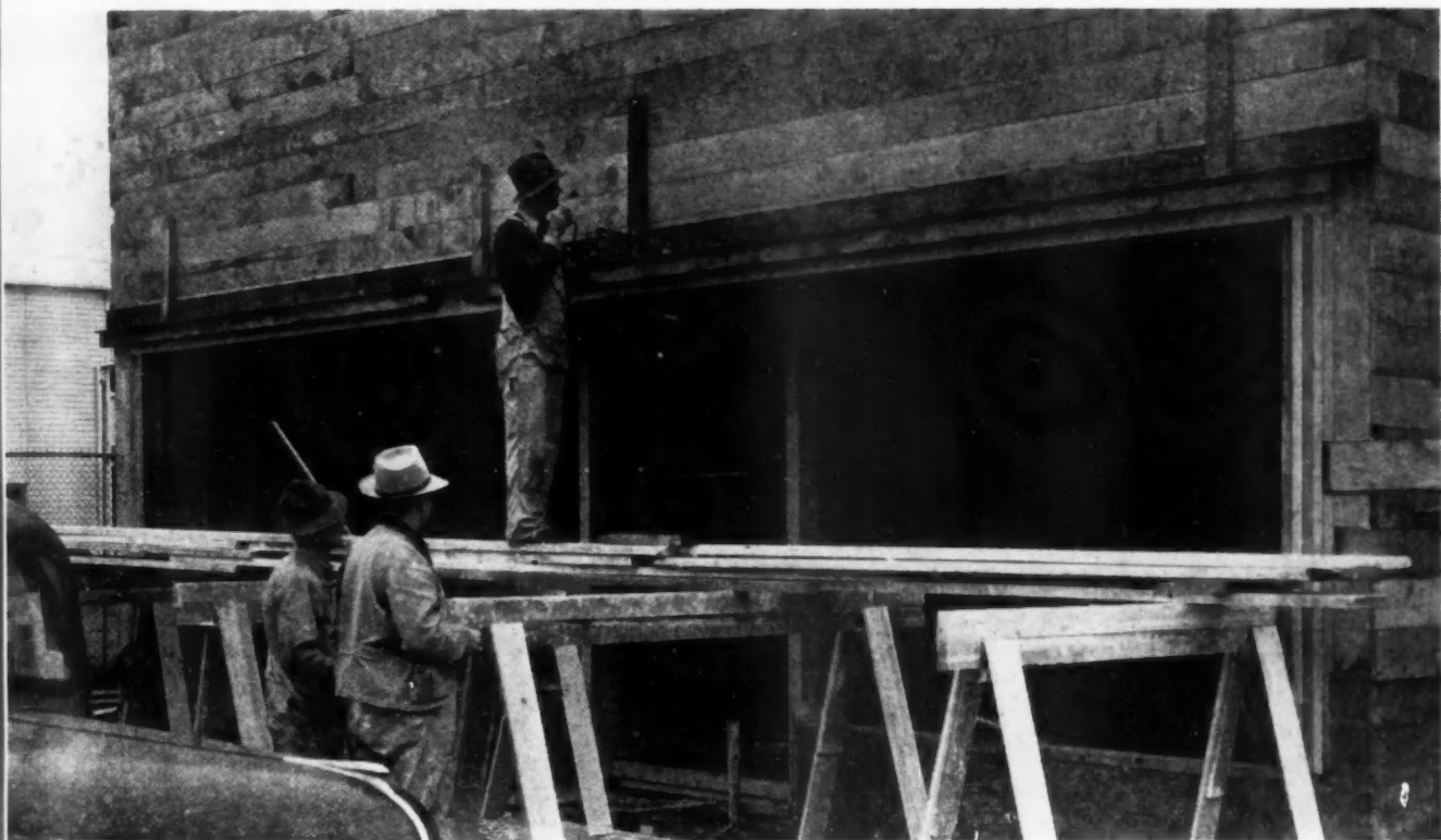
WORKMEN installing store front on extension to useless old shop in a Seattle suburb.
