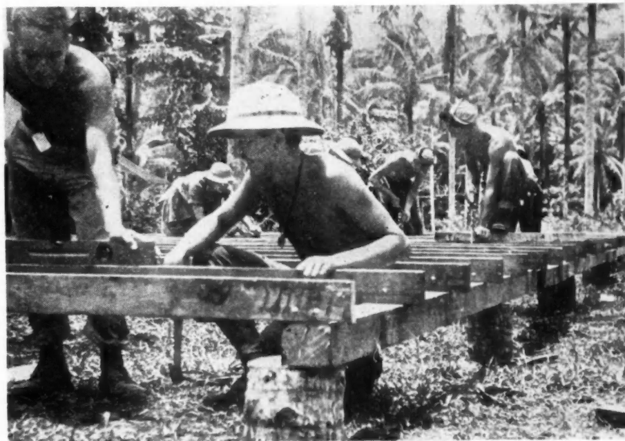
THEY WORK and fight —Seabees on newly captured Pacific island lay hospital foundation floor. Lumber was cut on spot with portable saw mills, brought in by marines.
