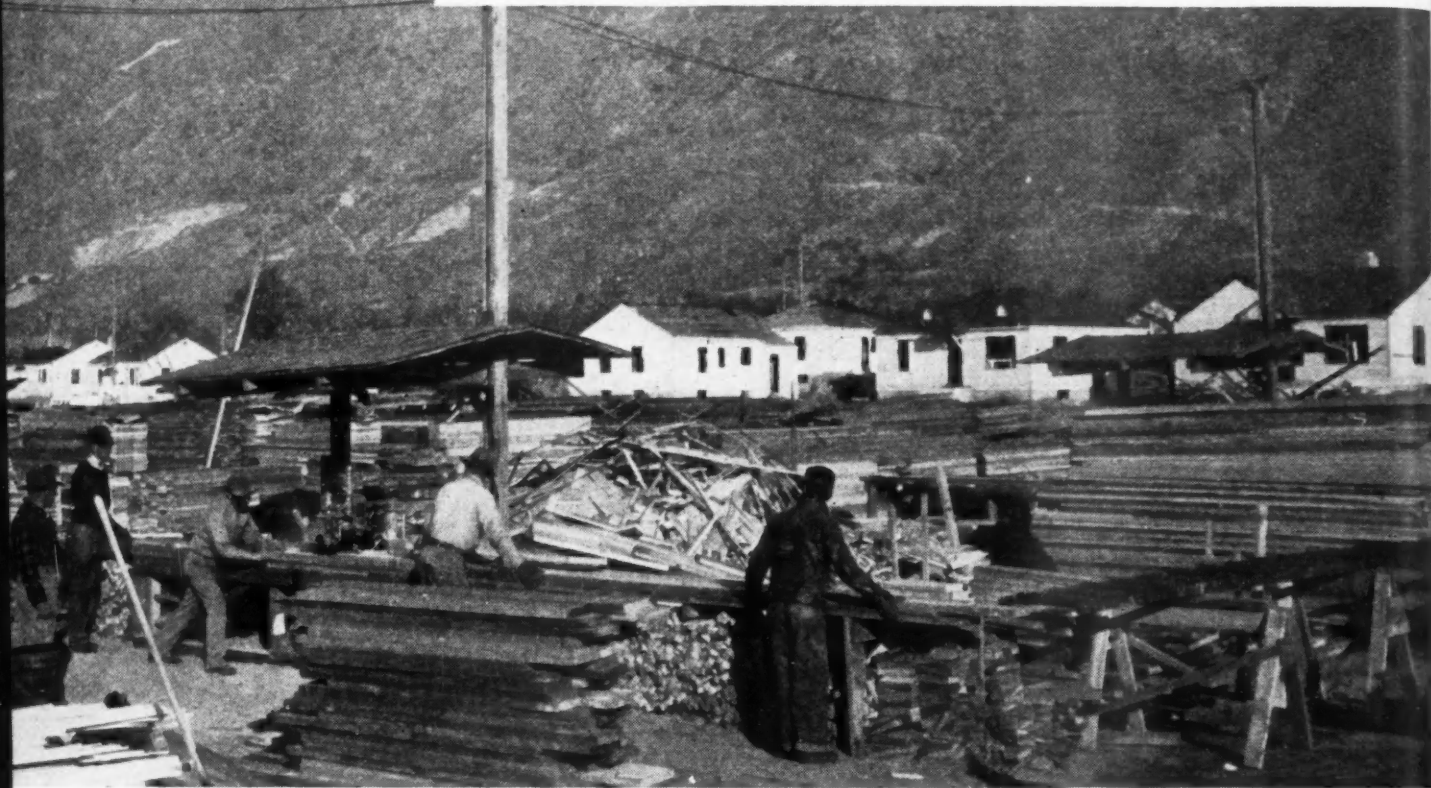
IN THE shadows of the Wasatch mountains Haddock Construction Co. precut all lumber for 172-house FHA Title VI project. Gable ends, door and window sections, and many other parts are prefabricated on the site, delivered by truck for quick erection. (See cover photos.)
