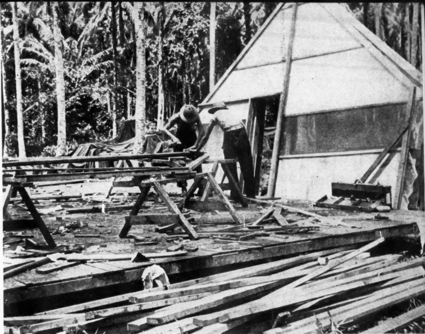
WITH LIVES at stake. Seabee carpenters break all records in constructing Marine hospital on jungle island in Southwest Pacific. The job was done practically under noses of Jap airmen soon after the island was captured.
